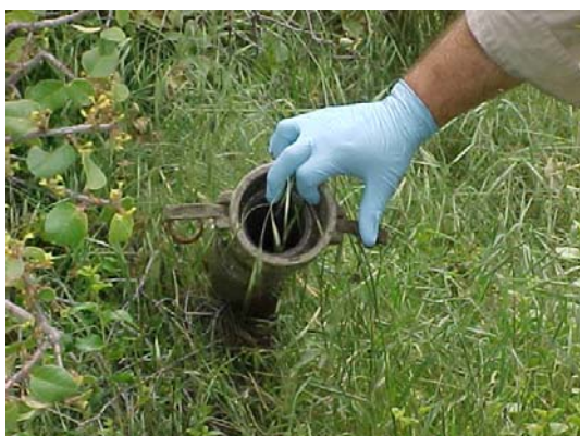
Photo 15. Beginning of flexible hose near Owens' well where evidence of septic discharge was found
