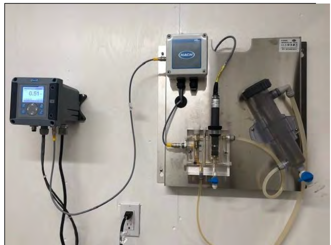
Figure 3.5: Chlorine disinfection system
