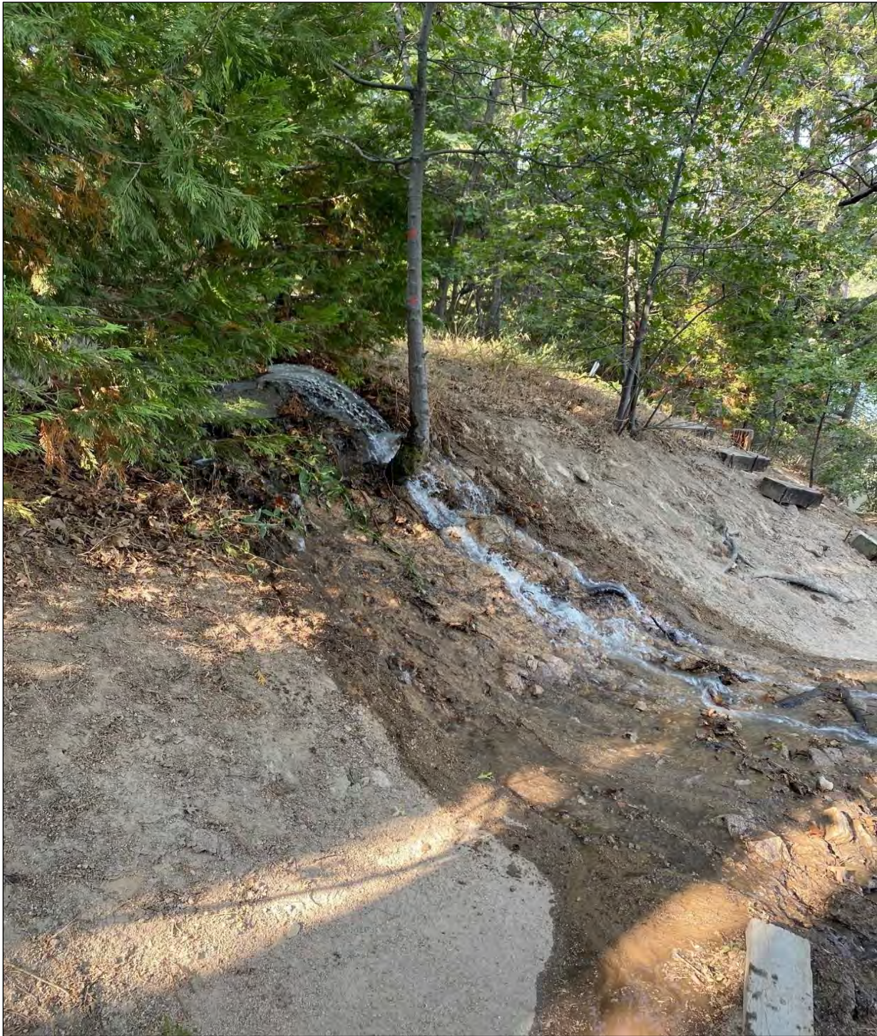
Figure 5.3 – Photograph of a July 2021, 2,900-gallon sewer line spill into Lake Arrowhead caused by blockage in the line.
