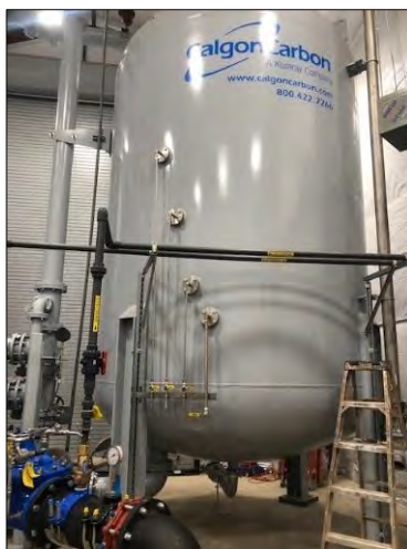
Figure 3.4: One of the two carbon vessels
