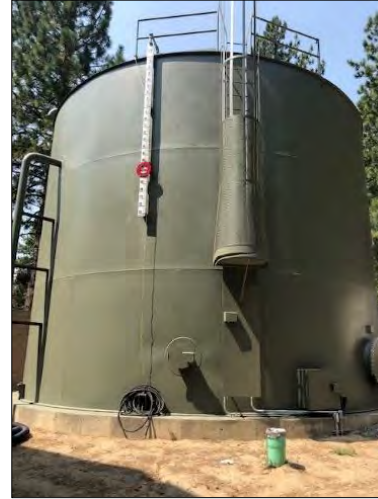
Figure 3.7: Treated water storage tank
