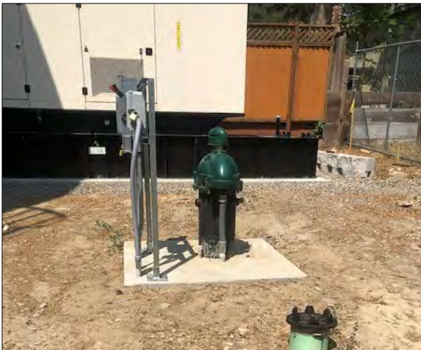
Figure 3.2: LBWC #5 and backup diesel generator
