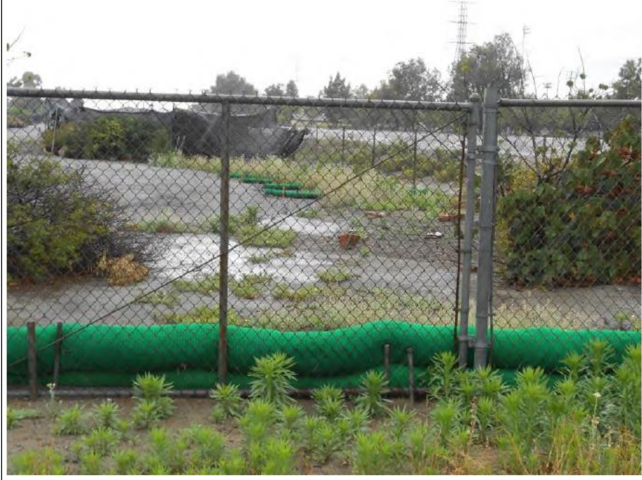
Figure 35 Filter Sox installed at San Gabriel River Nursery retains stormwater runoff from site
