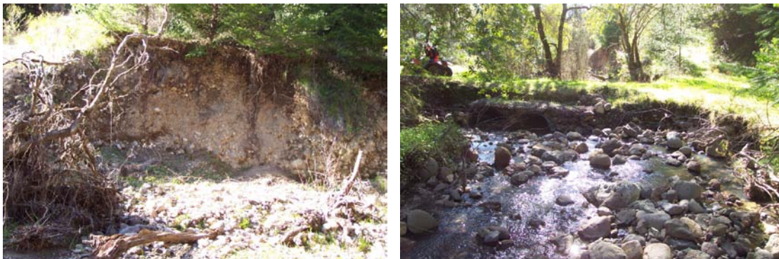
Figure 1. Example of an eroding bank of a headwater stream in the Pepperwood Preserve (left) and poorly designed stream culvert systems (right).
