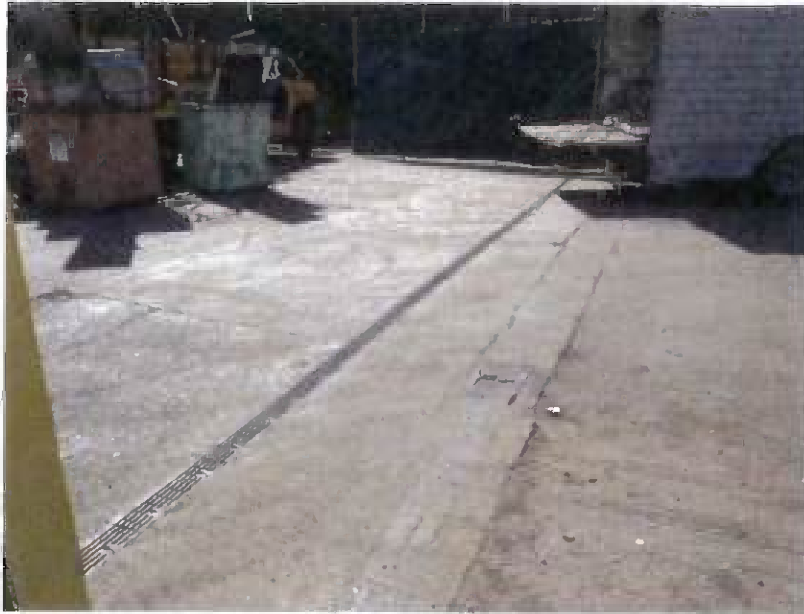
New strip drain to prevent off-site flow of stormwater at retail non-ferrous department entrance. Project completed – May 2012.
