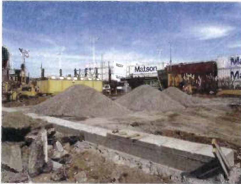
Grading, base preparation and footing construction underway to install additional tent structure to expand covered maintenance area. Expected project completion – October 31, 2012.
