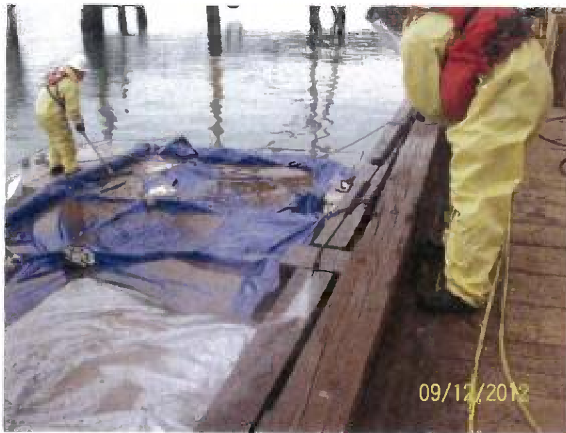
Dock cleaning activities. All wash water was captured by containment barge, profiled and disposed off-site. Dock cleanup activities completed September 6-14, 2012.
