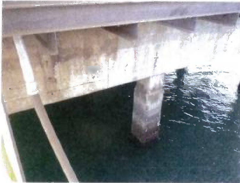
Demonstration of dock cleanup effectiveness. Dock face in right portion of photo has been cleaned. Dock cleanup activities completed September 6-14, 2012.
