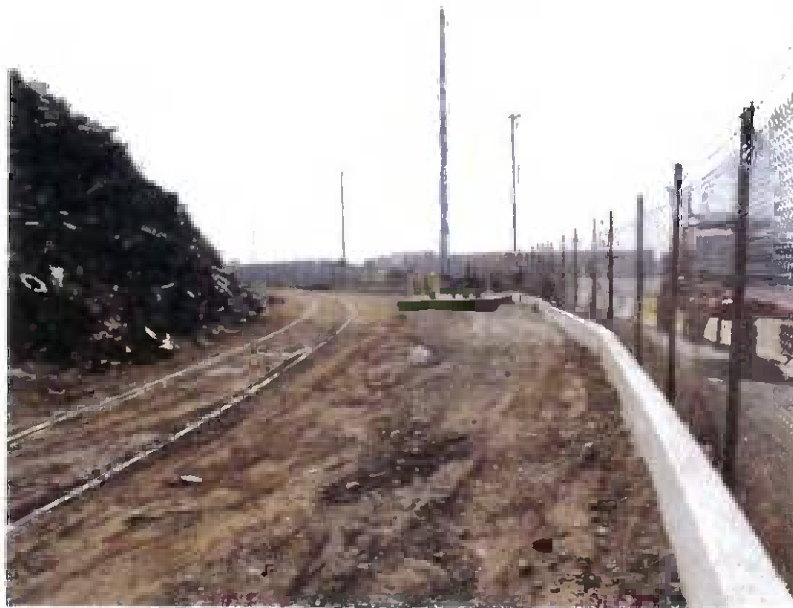
New extension of concrete containment wall along southwestern facility boundary. Over 600 lineal feet of new containment installed. Project completed August 24, 2012.
