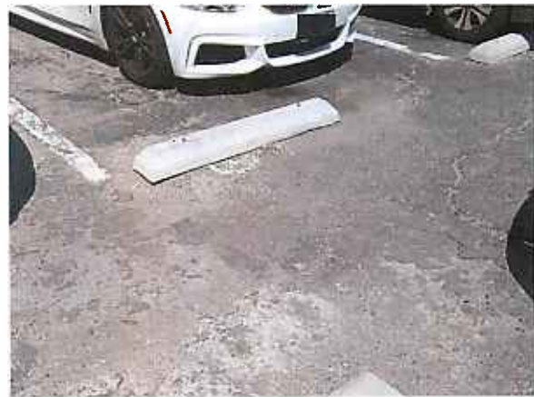
FIGURE 2 – Possible former drywell location in southern area of parking lot, with an unidentified cover underneath a parking block (Pit 4).
