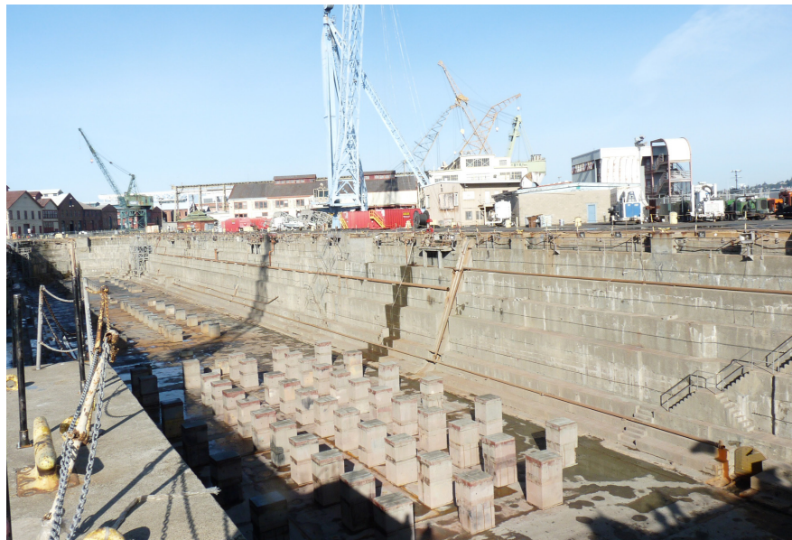
Photo below: Dry docks at Mare Island, covered under the Dry Docks NPDES general permit
