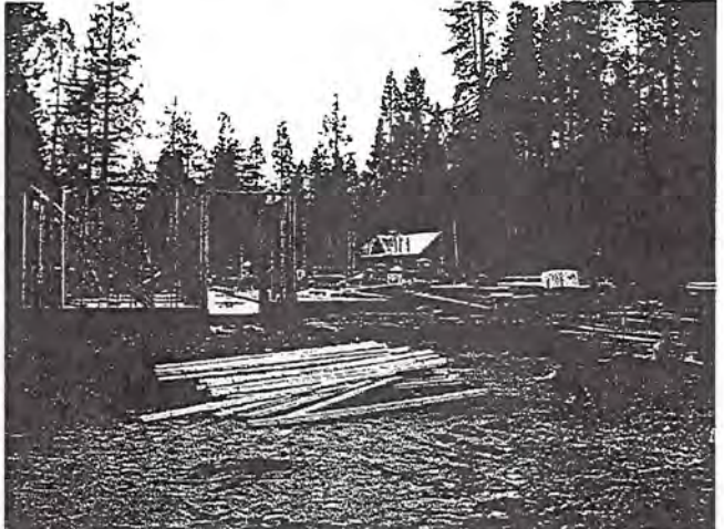
Photo 16. View of the construction area without erosion controls.
