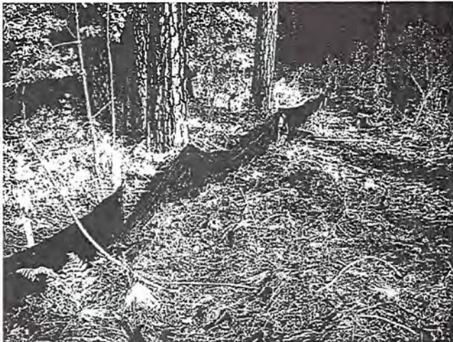
Photo 19. Unmaintained silt fence along the perimeter of the site.
