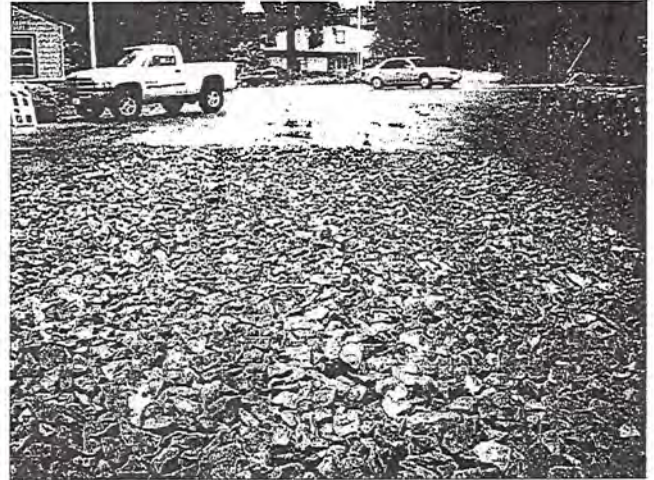
Photo 2. View of the construction entrance on 5 October 2011 with tracking onto Ridge Road.
