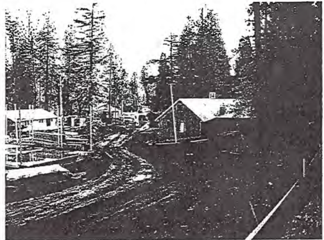
Photo 8. View of the access road looking towards the construction entrance. Unstabilized slope in foreground.
