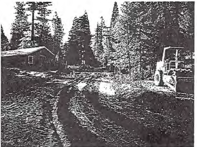
Photo 18. Saturated soils on the access road.
