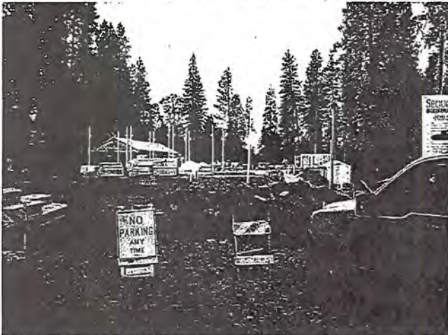
Photo 3. View of the constr. entrance at Ridge Road. The rock is not adequate to remove saturated soils from vehicle tires.
