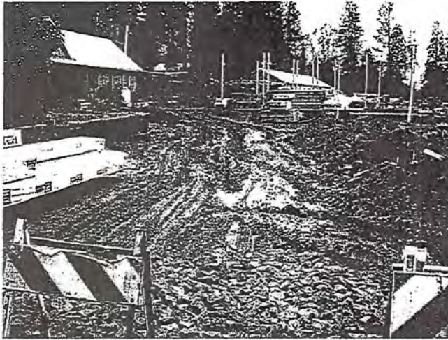
Photo 1. View of the construction entrance off Ridge Road on 5 October 2011. Saturated soils observed on site.
