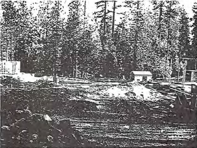
Photo 15. View of the construction area without erosion controls.
