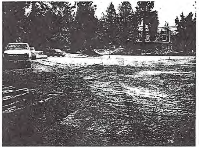
Photo 6. View of tracking from the construction site onto Ridge Road.
