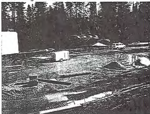
Photo 11. View of the construction area downhill from the Maintenance Garage. No erosion controls installed.
