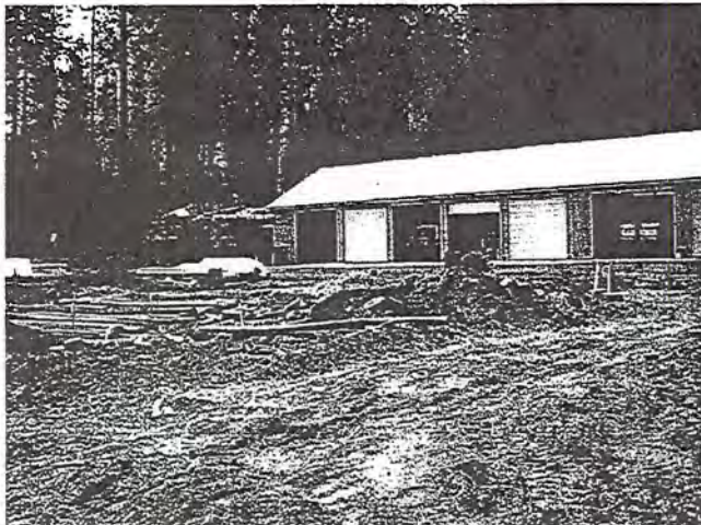
Photo 9. View of the Cal Fire Maintenance Garage that is active during construction. No erosion controls installed.
