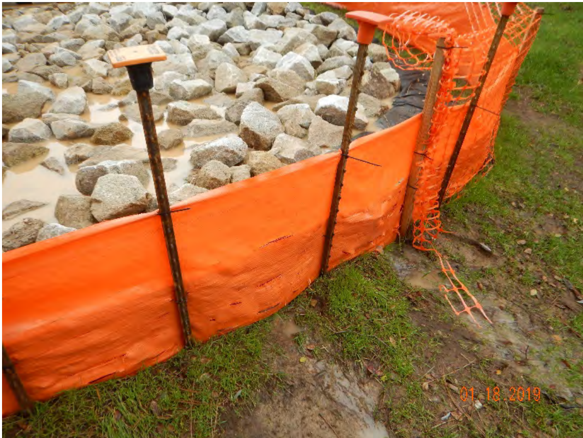
Photo 8. Tears in the silt fence allowing water to discharge.
