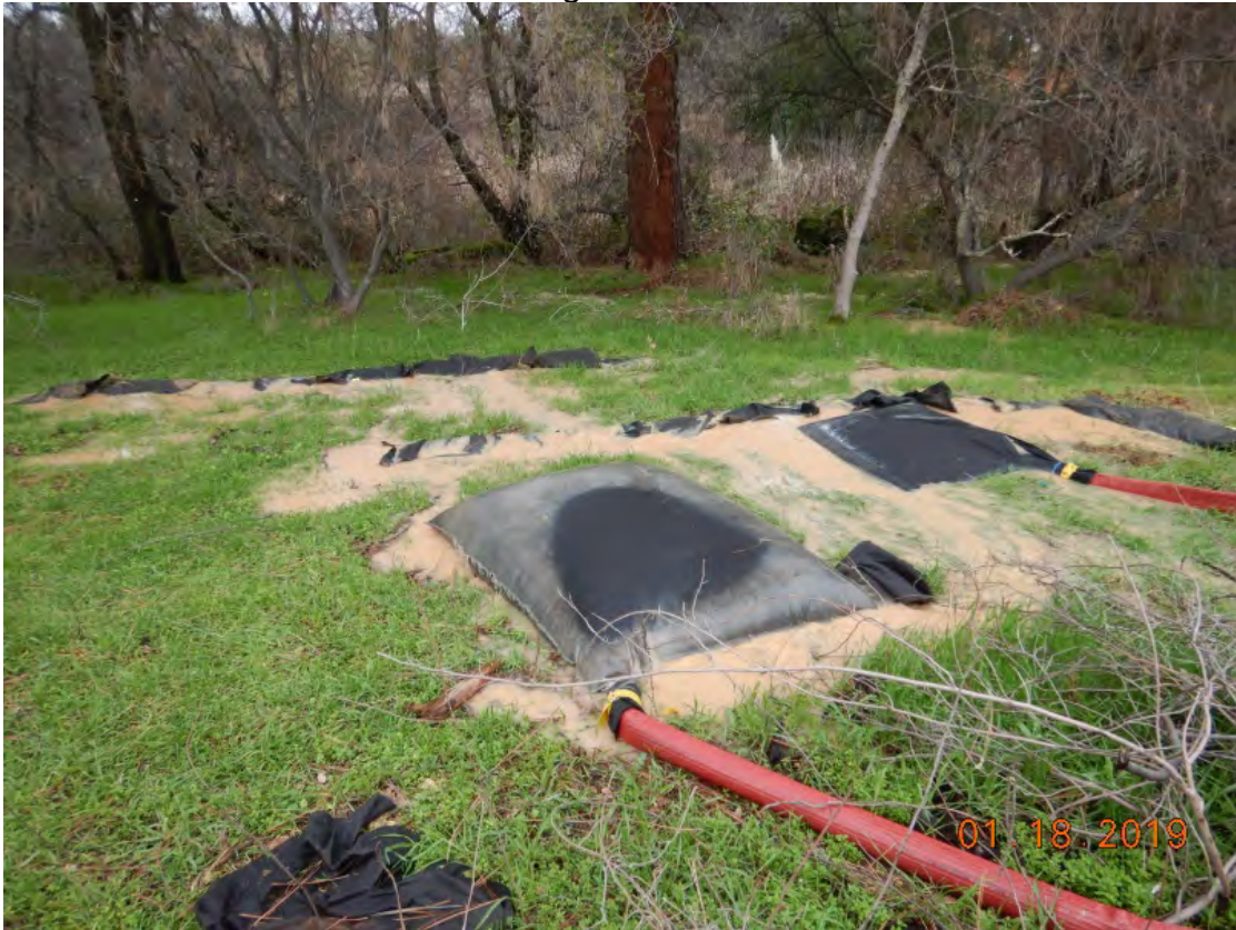
Photo 3. Filter bags and dewatering discharges from Project approximately 20 feet from a tributary to Secret Ravine.
