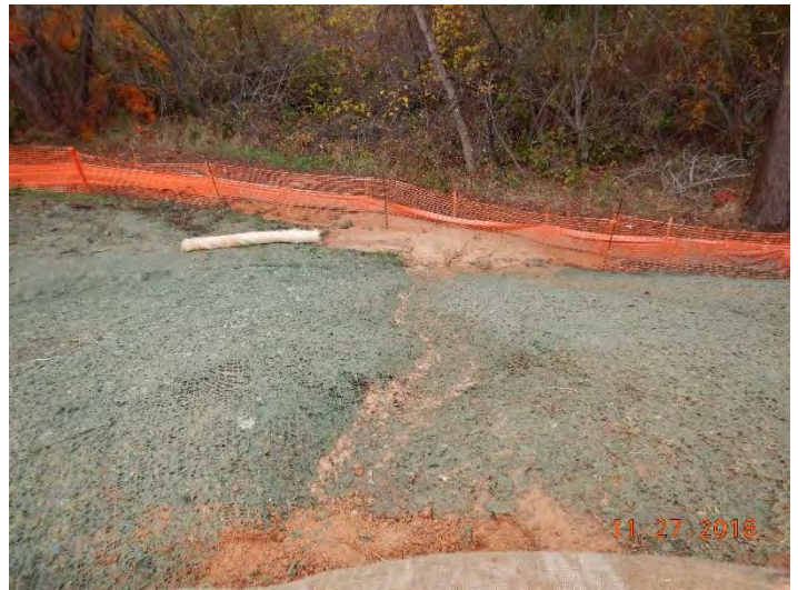
Photo 4. Silt fence in need of maintenance.
