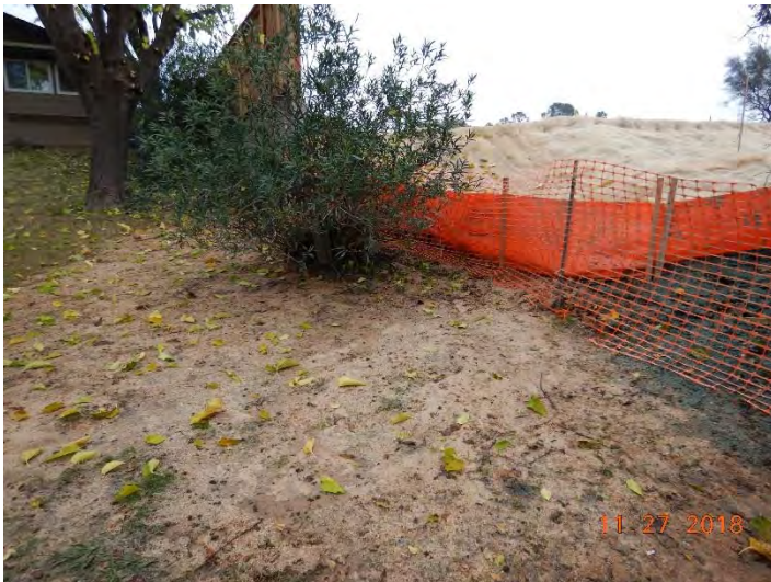
Photo 3. Evidence of sediment discharger from the Project.
