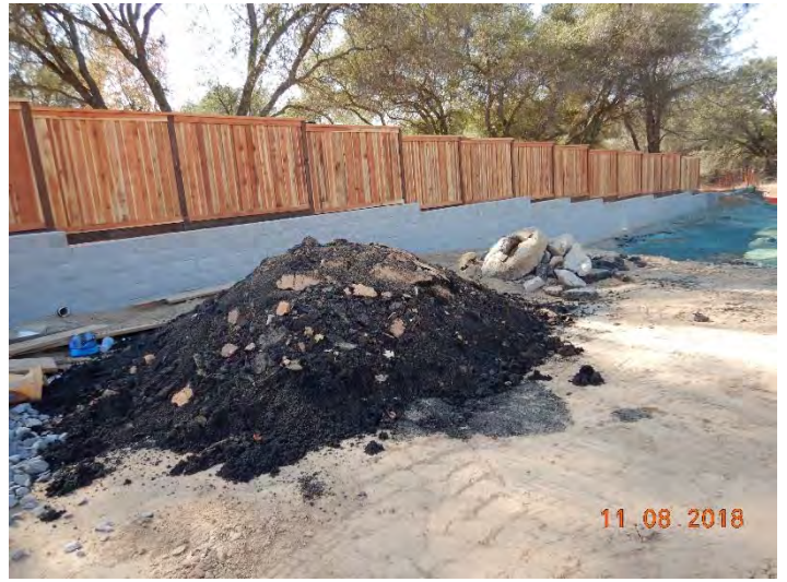
Photo 2. Asphaltic concrete not stored on permeable surface.
