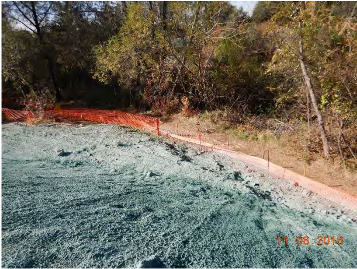
Photo 7. Damaged silt fence at Corona Circle lots.
