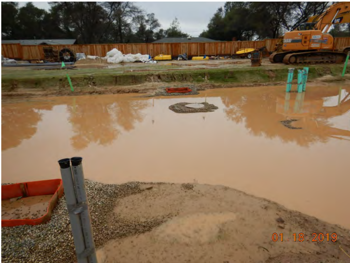
Photo 2. Road cuts accumulating water and entering the storm drain system.
