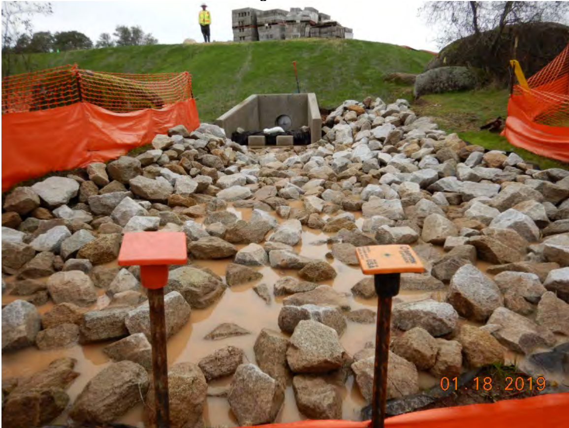
Photo 7. Water accumulating behind silt fence at storm drain outfall.
