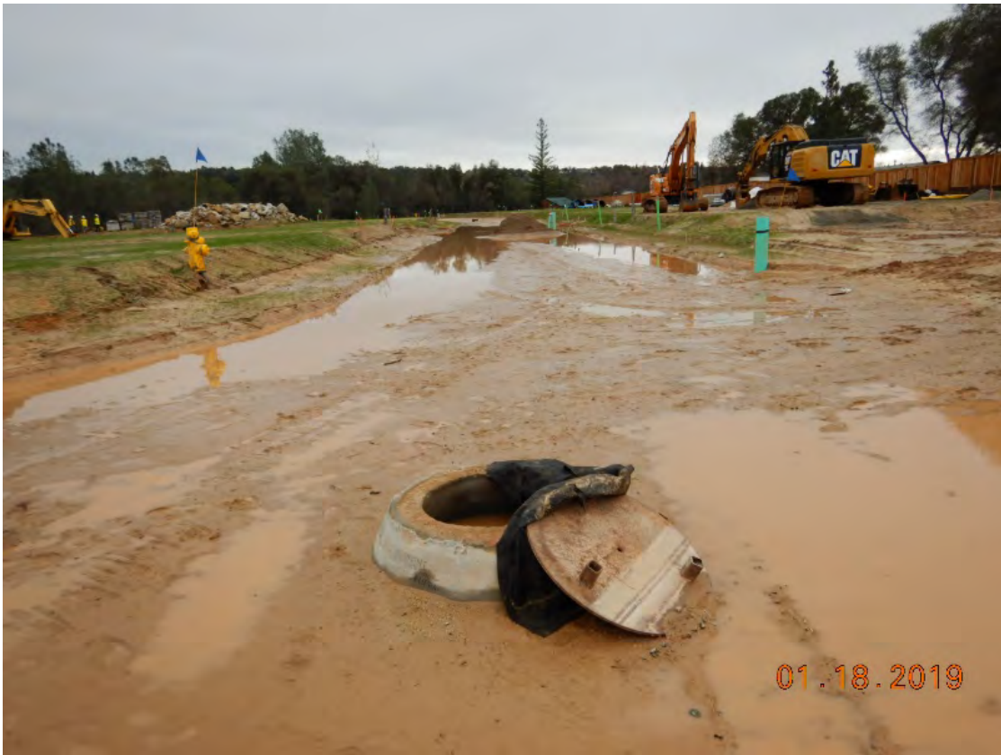
Photo 1. No erosion control was applied on road cuts.
