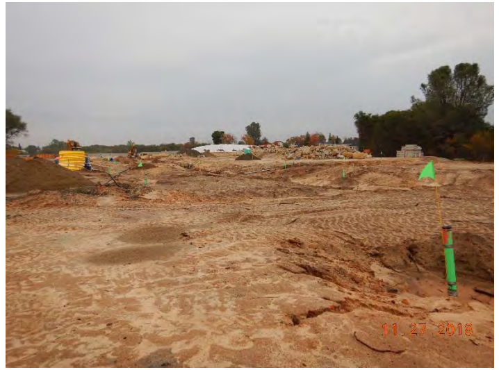
Photo 2. Open area without erosion control BMPs during a storm event.
