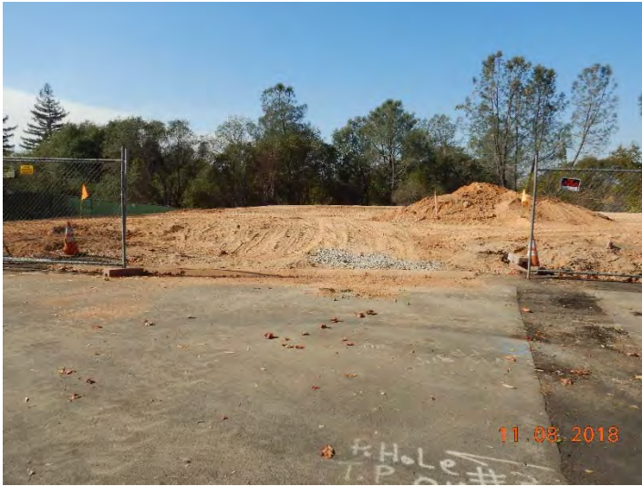
Photo 1. Missing construction entrance and tracking
