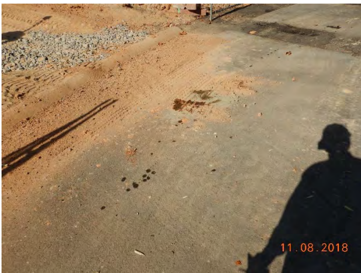
Photo 5. Oil spill on ground at Corona Circle.
