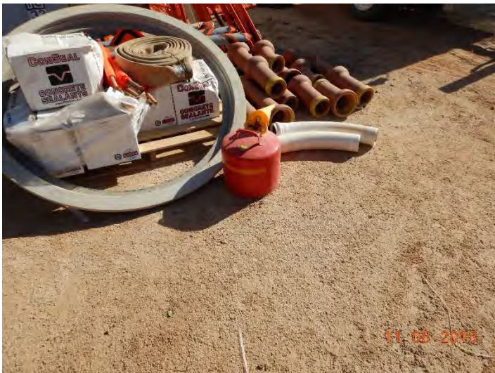
Photo 3. Gas can container outside of secondary containment.
