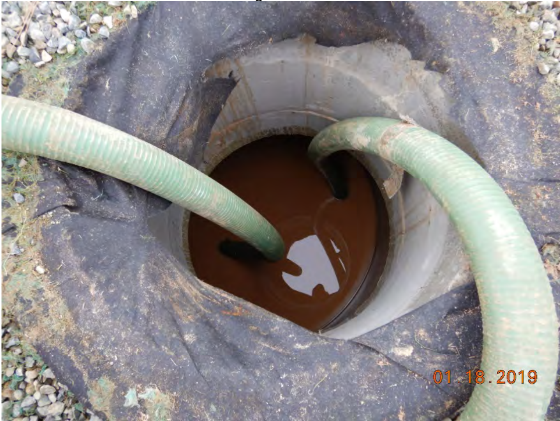
Photo 5. Dewatering hoses exiting the storm drain manhole leading to the pump and filter bags shown in Photo 3.
