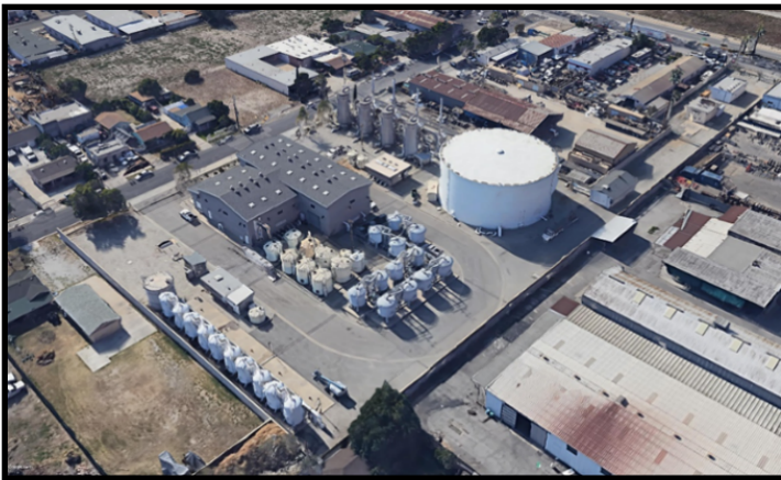
Figure 4. Valley County Water District's Lante Treatment Plant uses multiple treatment processes to address contaminants in groundwater
