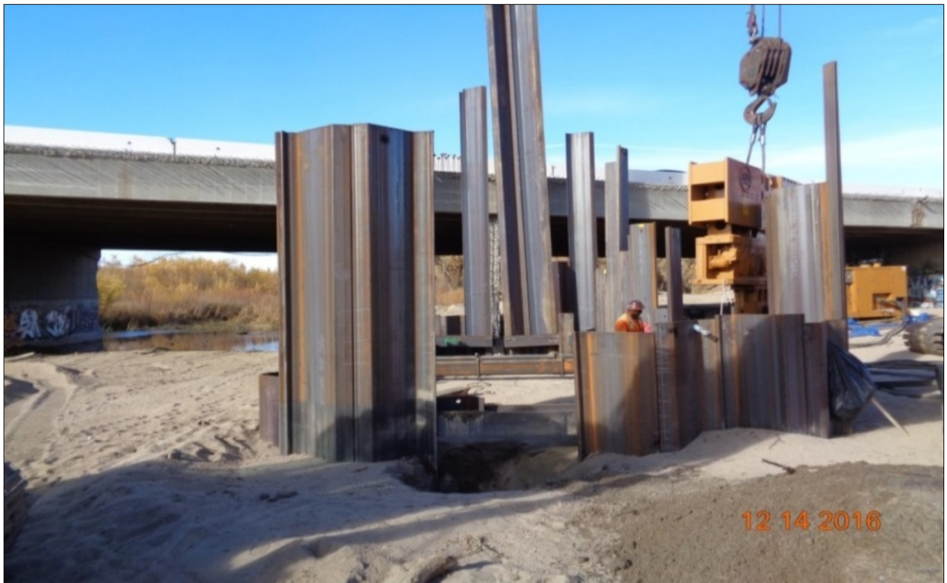
Installation of the first cofferdam using interlocking sheet piling at Pier #6 of the I-15 bridge
