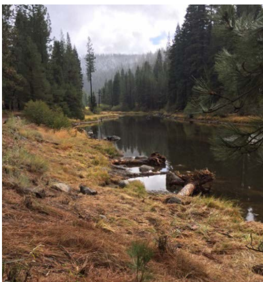
Truckee River Bank Stabilization Project by the Truckee River Watershed Council. One location showing a previously eroding vertical bank that had been filled and sloped with rocks, logs with roots attached, and gravel
