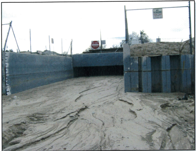
Photo 2 – View looking upstream at the Oro Grande Box where it discharges to the Mojave River. The box is 12-foot by 12-foot; nearly 7-feet of sediment was deposited following a single rain event during December 2015.
