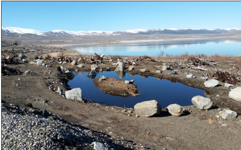
Figure 2 – Post Office Creek flow was diverted into an old, historically constructed channel and pond on the property, and wood and other debris was cleared and stockpiled on the site.
