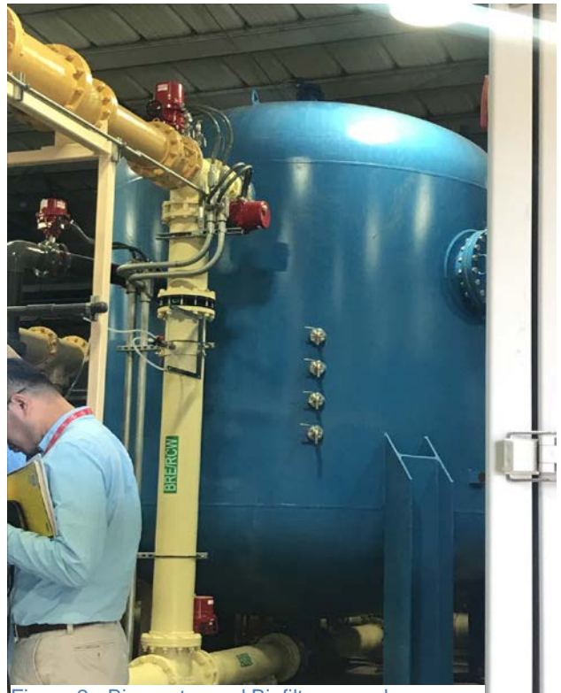
Figure 2 - Bioreactor and Biofilter vessels
