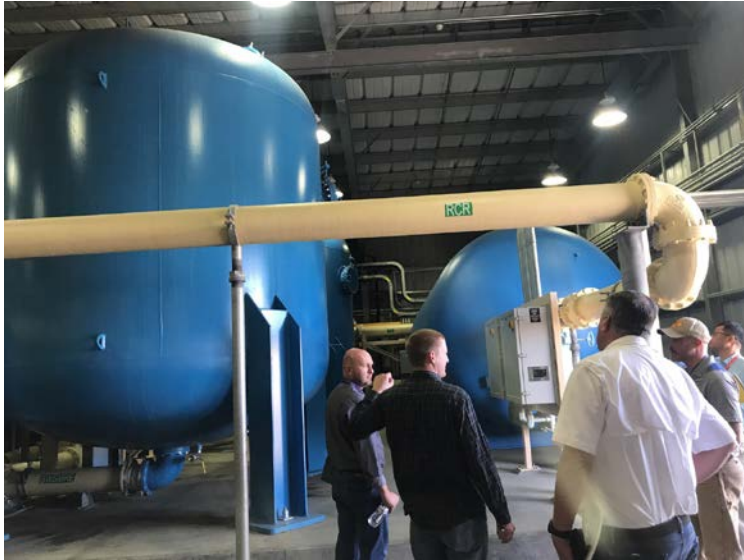
Figure 3 - Final vessel for removing suspended solids and high turbidity. Note sampling ports on the side of the vessel.
