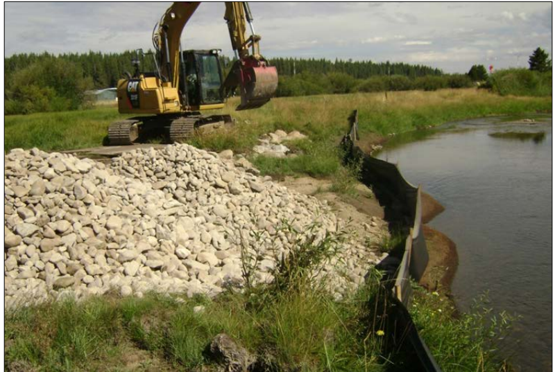
Photo 2: Bank repair work conducted in September 2017, as part of the Adaptive Management Plan.
