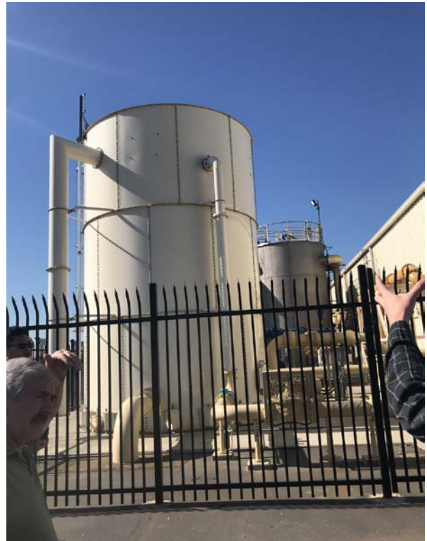
Figure 1 - Influent equalization tank at the head works of the facility
