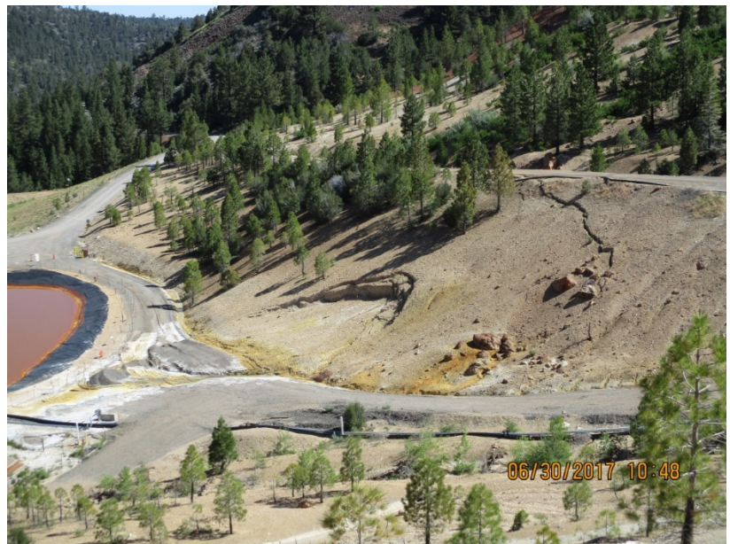
Figure 2 June 30, 2017 – Soil slump near Pond 4
