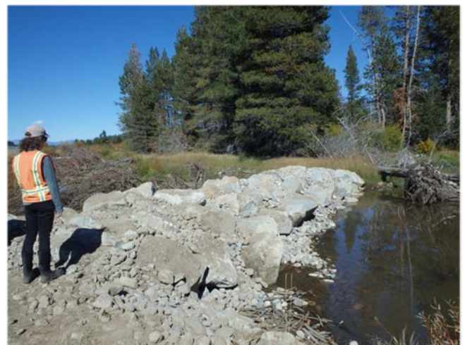
Photo 3: Rock check dam constructed in September 2017, as an emergency stabilization measure in the partially backfilled historic channel.
