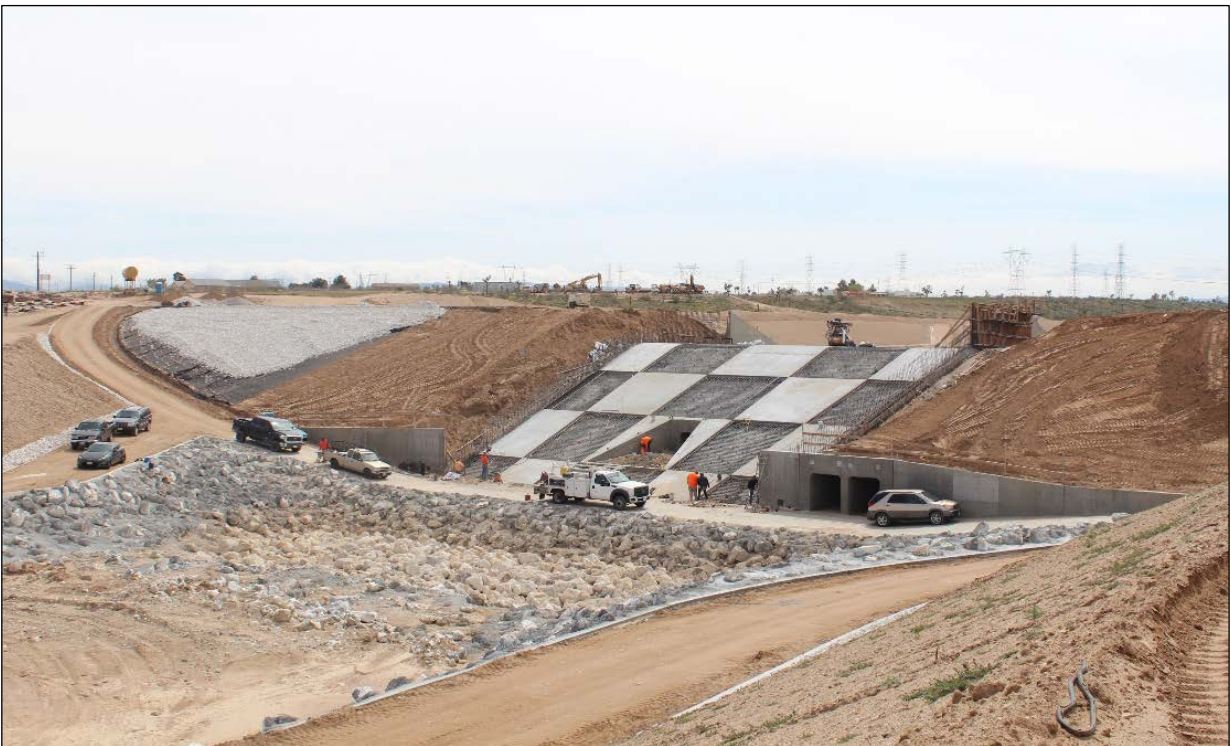
Figure 11b - View of the spillway still under construction and the two gated drain culverts
