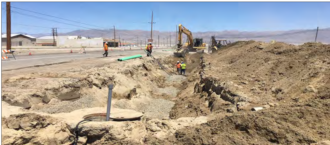
Figure 9.2 - View to north, along CA Highway 178, during replacement of failed collection system pipes.
