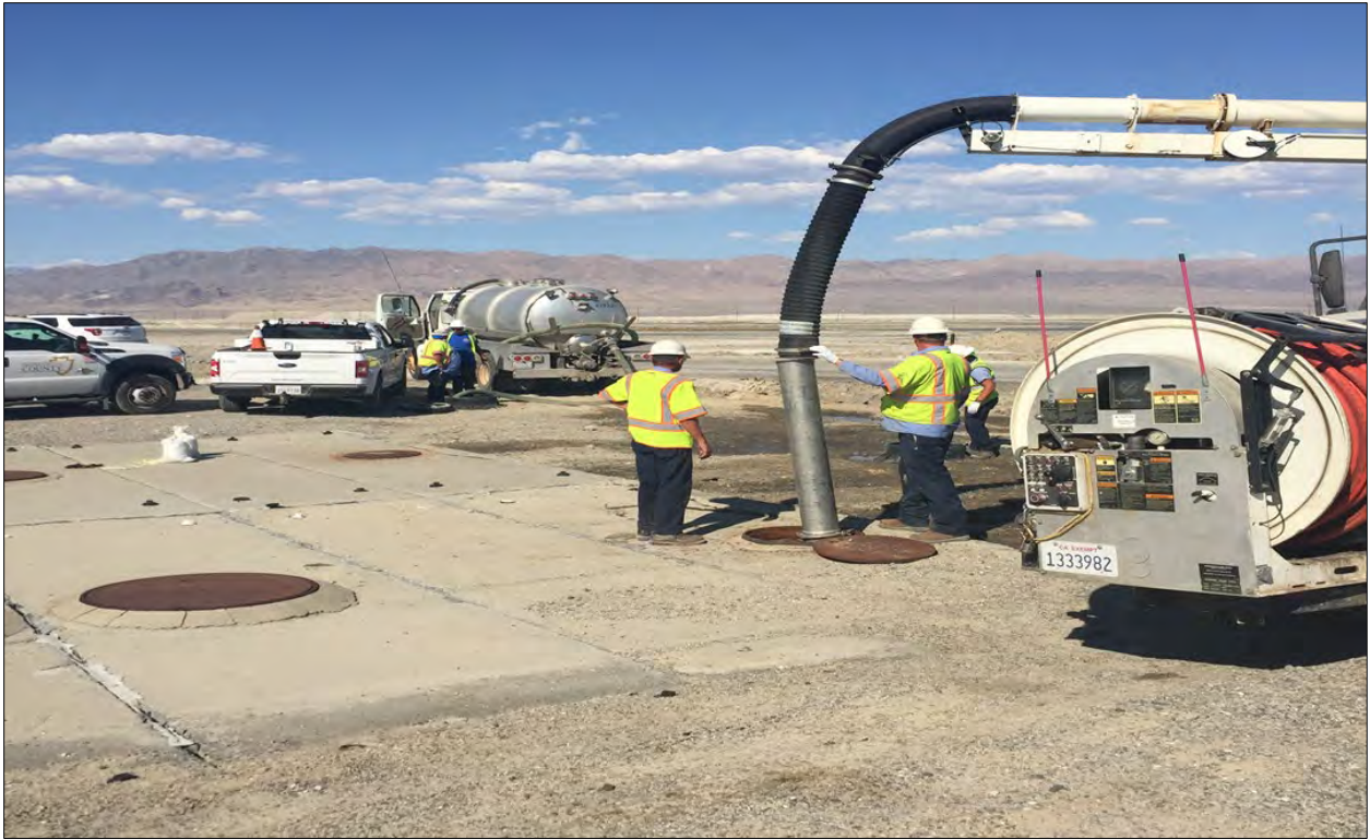
Figure 9.3 - View to east, main Trona septic tanks are pumped, cleaned, and inspected. Removed septage was disposed in the CSA 82 disposal ponds located on the east side of Searles Dry Lake.
