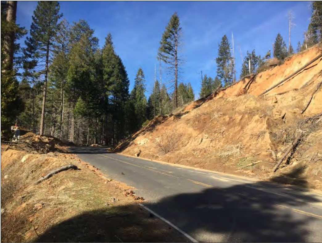
Figure 5.2 - Partially completed restoration of a landslide on a main timber access corridor. Hillside collapse occurred after a series of 2017 rain-on-snow events.
