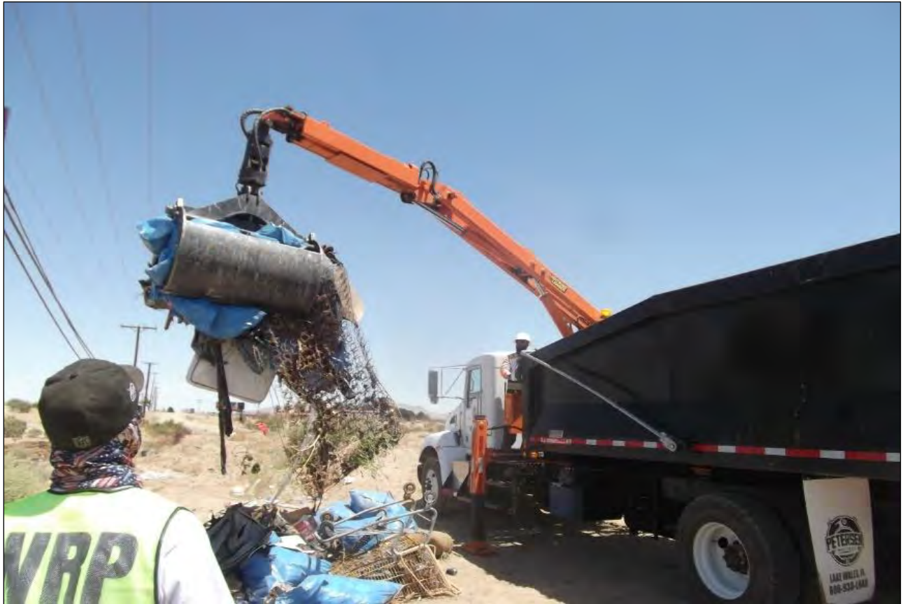
Photo 10.2 – Clam-shell crane scooping up debris found in Oro Grande Wash and placing debris new city-owned truck to haul offsite for disposal.
