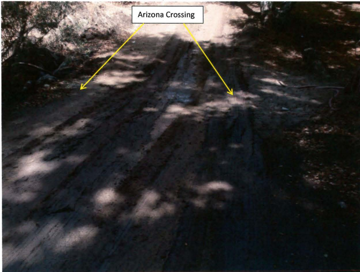
Photo 32. This photo shows an Arizona crossing in Ybarra Creek in Parcel 2821-009-023. This photo was taken near latitude: 34 18.158 and longitude:-118 36.665.
