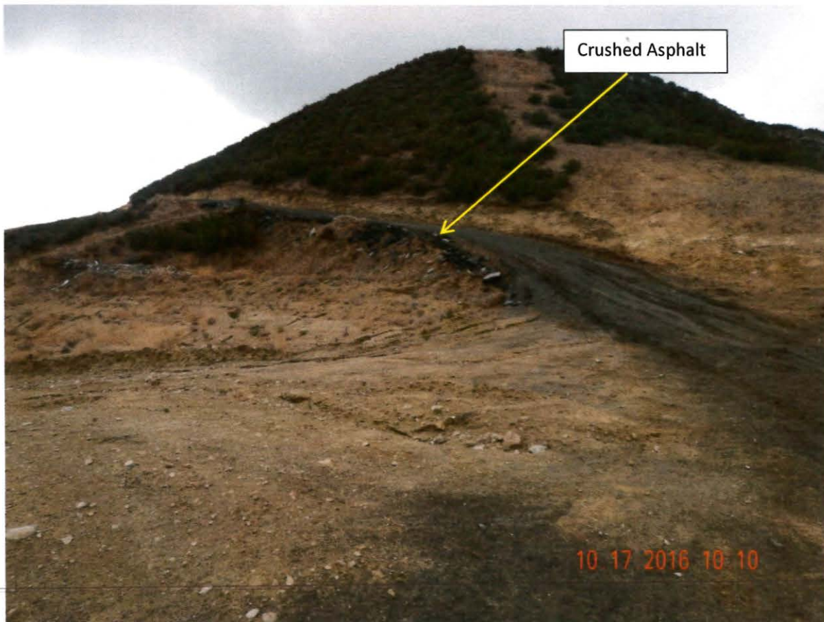
Photo 13. This photo shows crushed asphalt that was used to build the road. This photo was taken near latitude: 34 18.574 and longitude: -118 37.078 in Parcel 2821-002-025.
