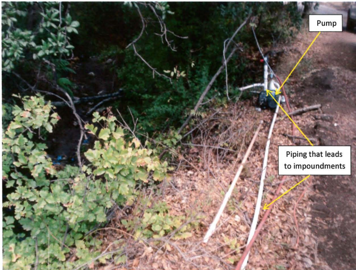
Photo 35. This photo shows the pipes in Photo 34 were connected to a pump. The pump was not in operation at the time of the inspection. This photo was taken in Parcel 2821-009-023 near latitude: 34 18.158 and longitude:-118 36.665.
