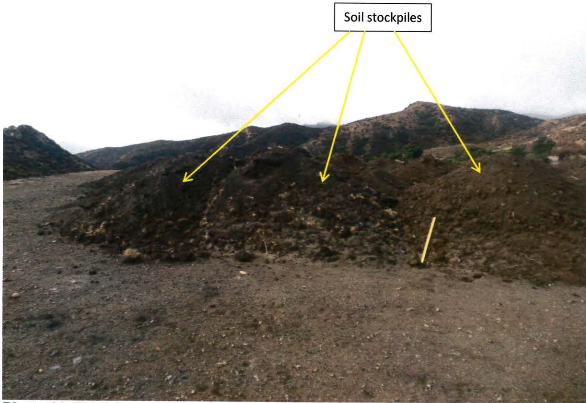
Photo 28. This photo shows stockpiles of soil found in Parcel 2821-009-031. This area lacked erosion or sediment control BMPs. This photo was taken near latitude: 34 18.264 and longitude -118 36.644.
