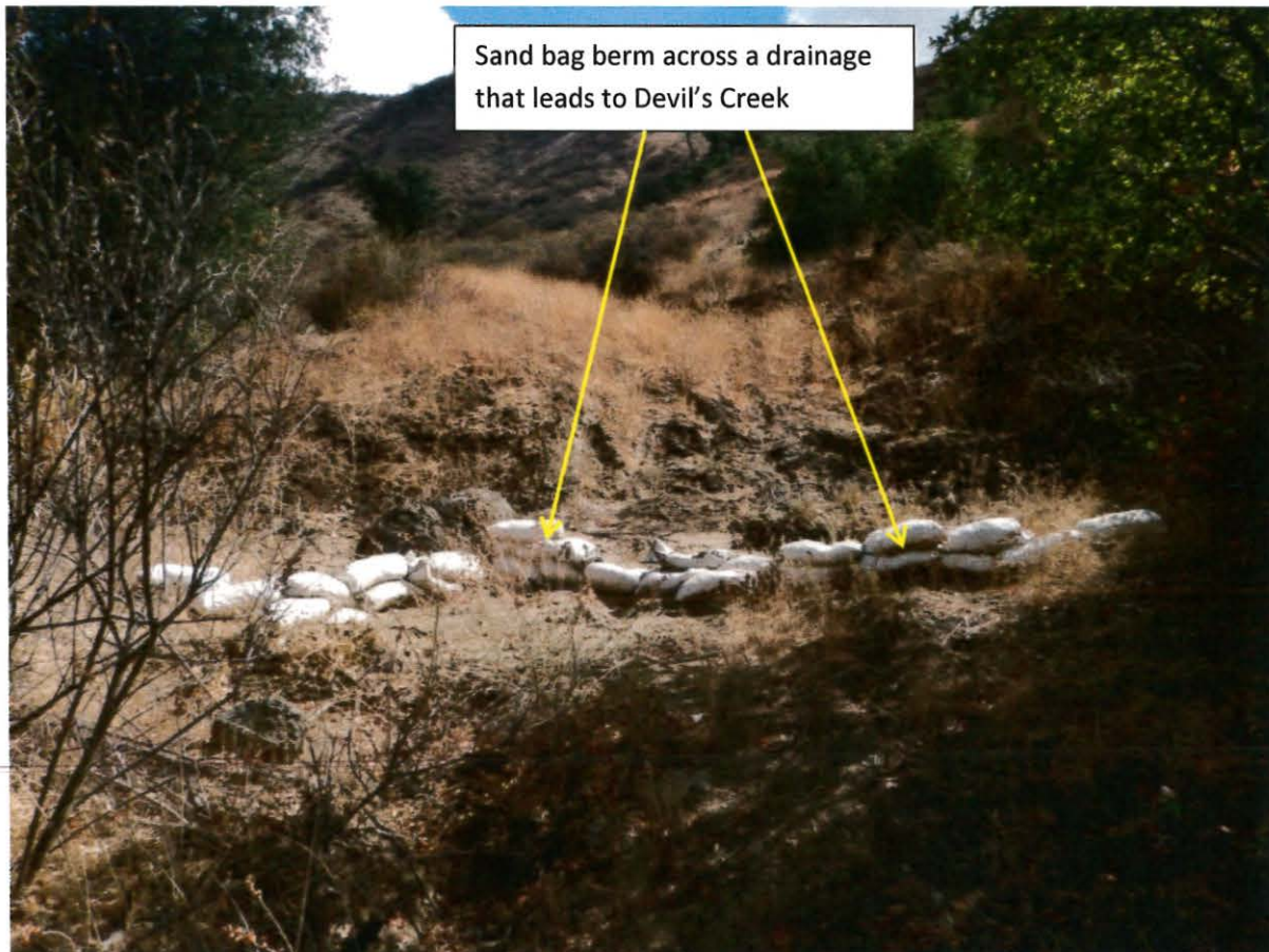
Photo 10. This photo shows another view of the sand bag berm located in a drainage that leads to of Devil's Creek. The sand bag berm shown is the same sand bag berm shown in Photo 8. This photo was taken on Parcel 2821-002-025, at latitude: 34 18.568 and longitude: -118 37.418.
