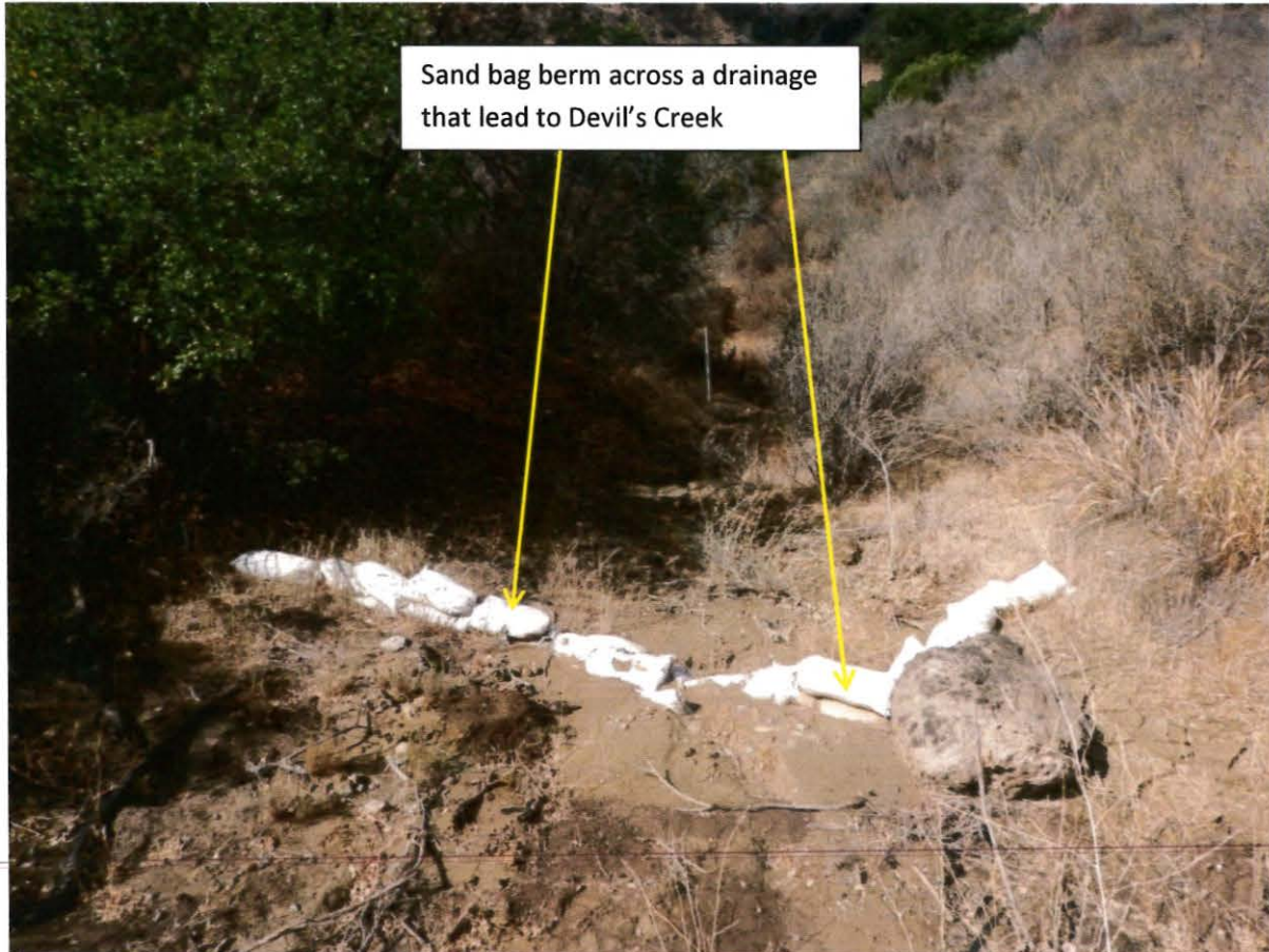
Photo 9. This photo shows a sand bag berm located in drainage that leads to Devil's Creek. This photo was taken on parcel 2821-002-025, at latitude: 34 18.568 and longitude: -118 37.358. This area lacked erosion control best management practices, and there was loose sediment accumulated behind the berm.
