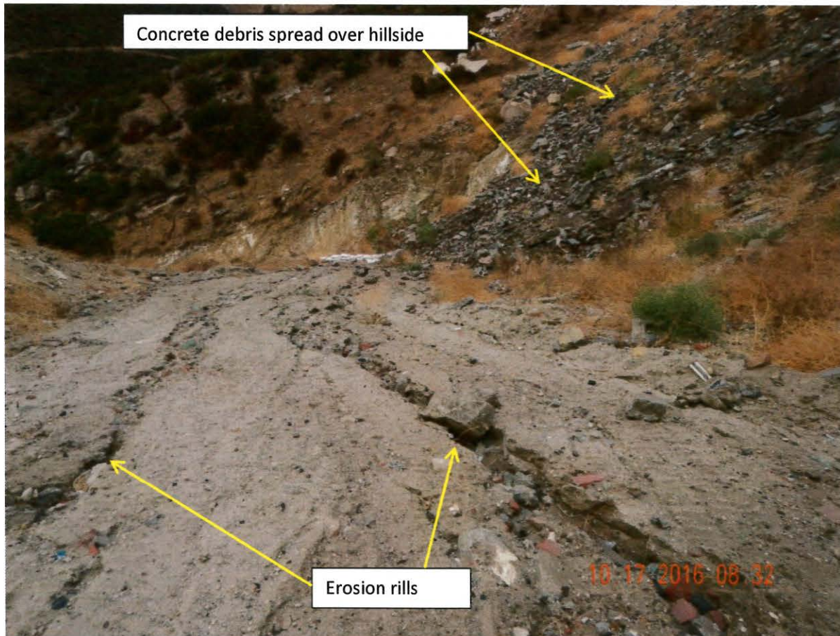
Photo 19. This photo shows erosion occurring on the road in Parcel 2821-002-023 above the sand bag dams. This photo was taken near latitude: 34 18.626 and longitude -118 36.767.
