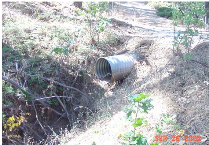
Figure 31. Example of an existing culvert with scour at the outlet for a central Sierra Nevada THP included in the MCR sample.
