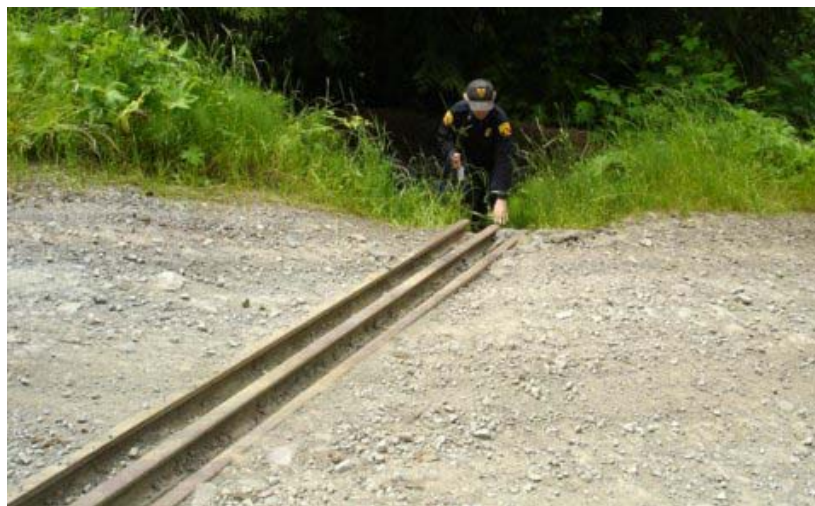
Figure 37. Pete Cafferata, CDF, points to the outlet of a uniquely-designed 3-rail cutoff-drainage structure on the approach to a watercourse crossing located in a forested watershed on the North Coast of California. Features like this, commonly a rolling dip without the rails, are used to prevent direct discharge of road runoff into watercourse channels.
