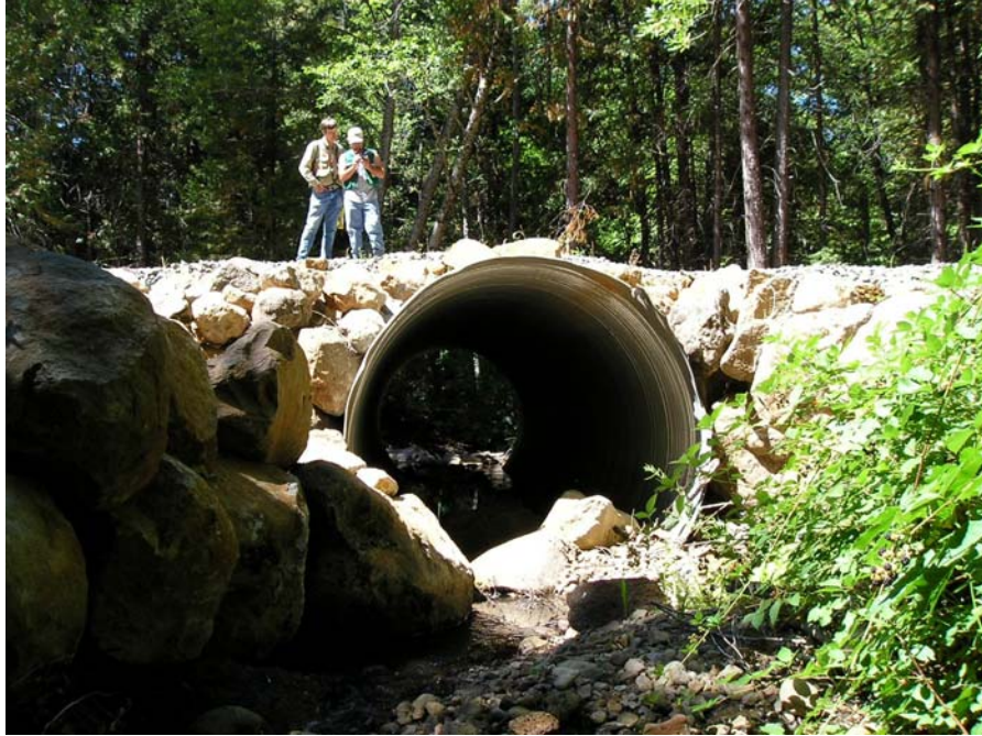
Figure 12. Pilot project Inland team members Dave Longstreth, CGS, and Joe Croteau, DFG, at a culvert installed on a THP in Shasta County in August 2006.
