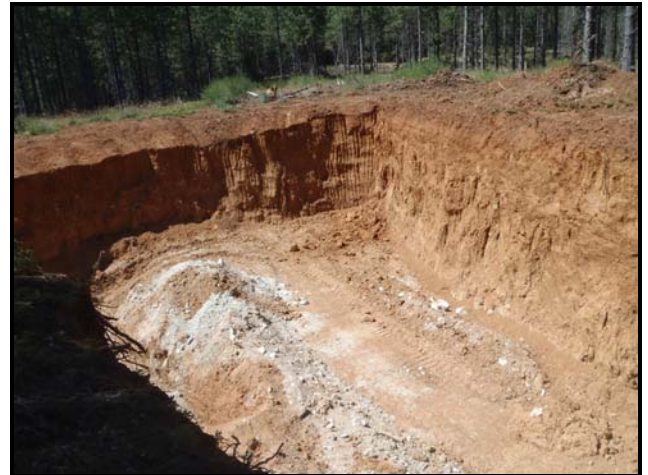
Photo 4. Newly excavated mining pit, dimensions are approximately 75-feet wide 100-feet long and 15-feet deep.
