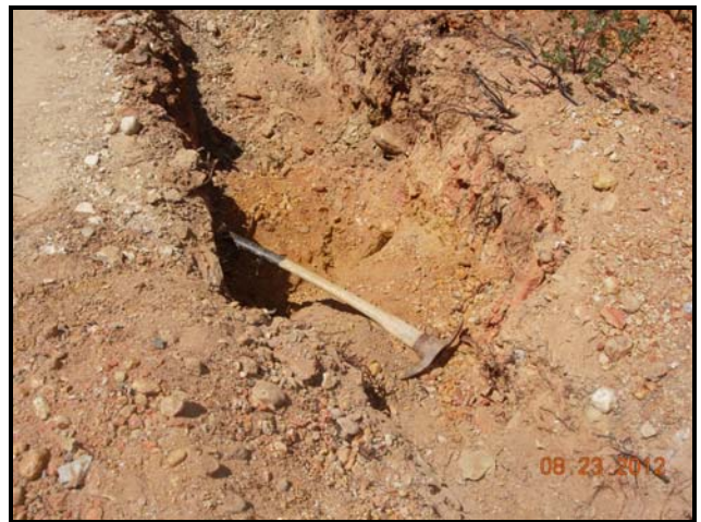
Photo 17. Very recent excavation of the bedrock, south east side of the old Hoffman Pit area.
