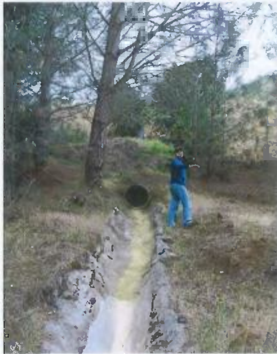
Photograph B-38: Storm water runoff outlet piping from upper mine workings area.
