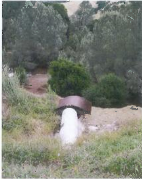
Photograph B-39: Storm water runoff outlet piping from upper mine workings area.
