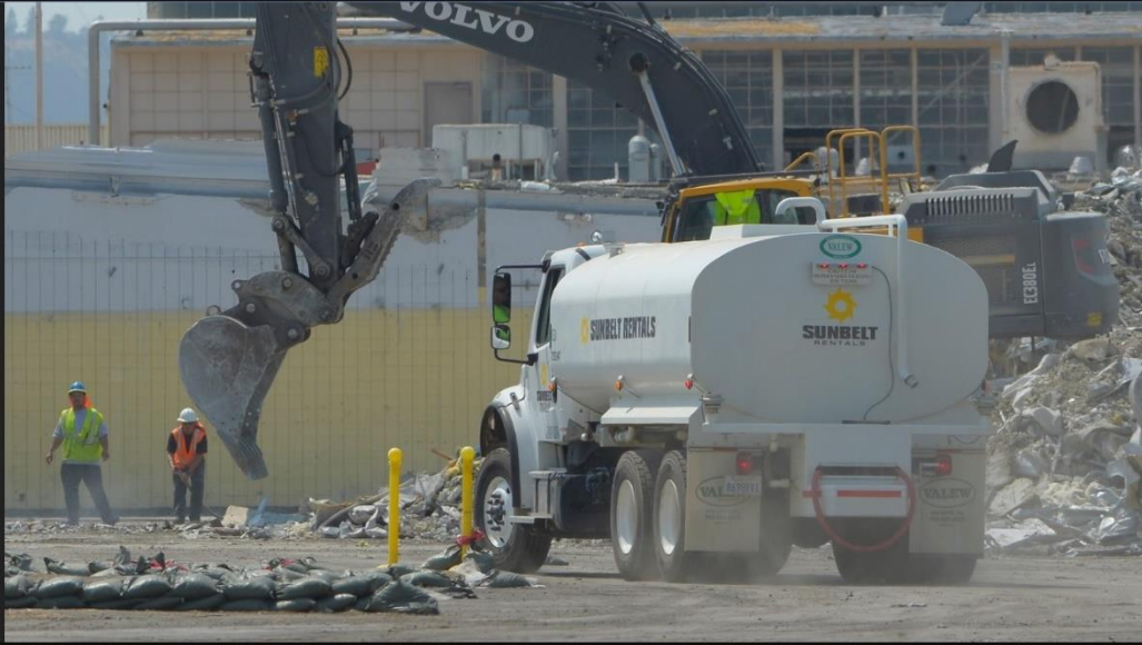
Rocketdyne was a rocket engine manufacturing plant that began in 1955. Buildings at the site contain some asbestos, and soil at the site has to be cleaned of the chemicals associated with the manufacturing process. The site is being razed for development. Canoga Park, CA. August 24, 2016. (Photo by John McCoy/So Cal News Group)
