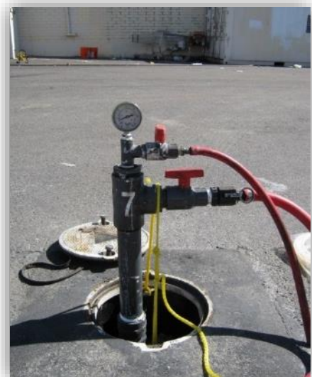
Photo by: Nick Amini, Santa Ana Regional Water Board staff.
