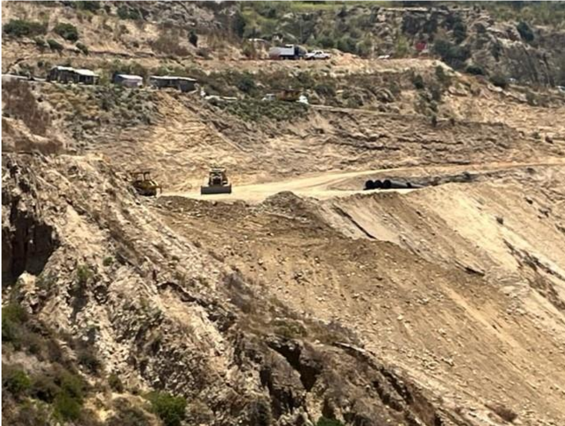
Figure 3: Materials stockpiled in Matadero Cañon for repair of PB1A (Source: IBWC).
