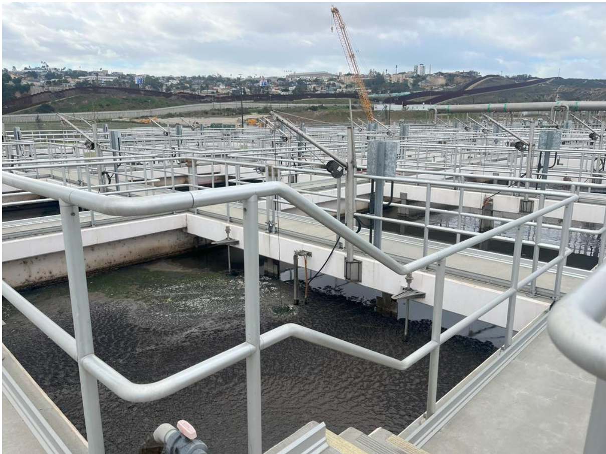
Figure 8: Secondary aeration tank. (MC 01/10/2024)
