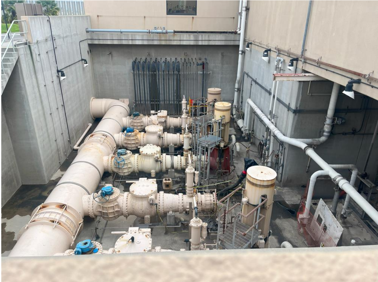
Figure 2: Influent pumps. (MC 01/10/2024)
