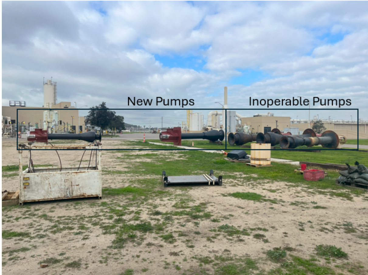
Figure 3: Two new influent pumps on the left. Three inoperable influent pumps on the right that have been removed for replacement. (MC 01/10/2024)
