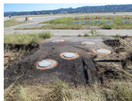
Photo 3. Junction Boxes and Soil Saturated with Jet Fuel - Further Cleanup Being Evaluated
