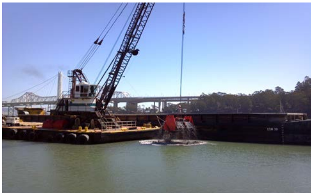
Photo 1a. Dredging at Clipper Cove. East span of the Bay Bridge and Yerba Buena Island are seen in the background. Photo taken September 17, 2013.
