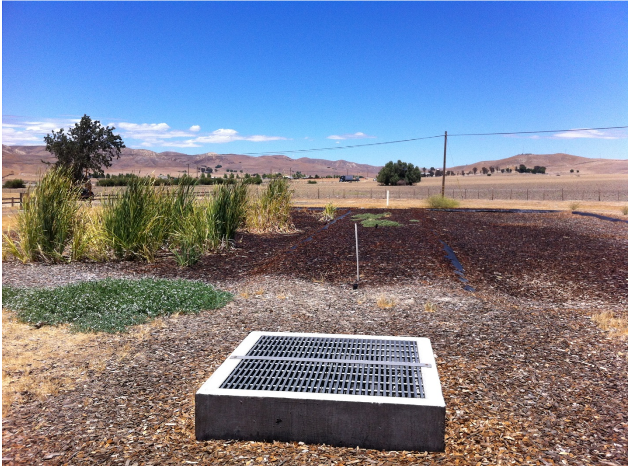
Figure 3 Photo taken of a woodchip bioreactor installed at a rest stop in Shandon California.
