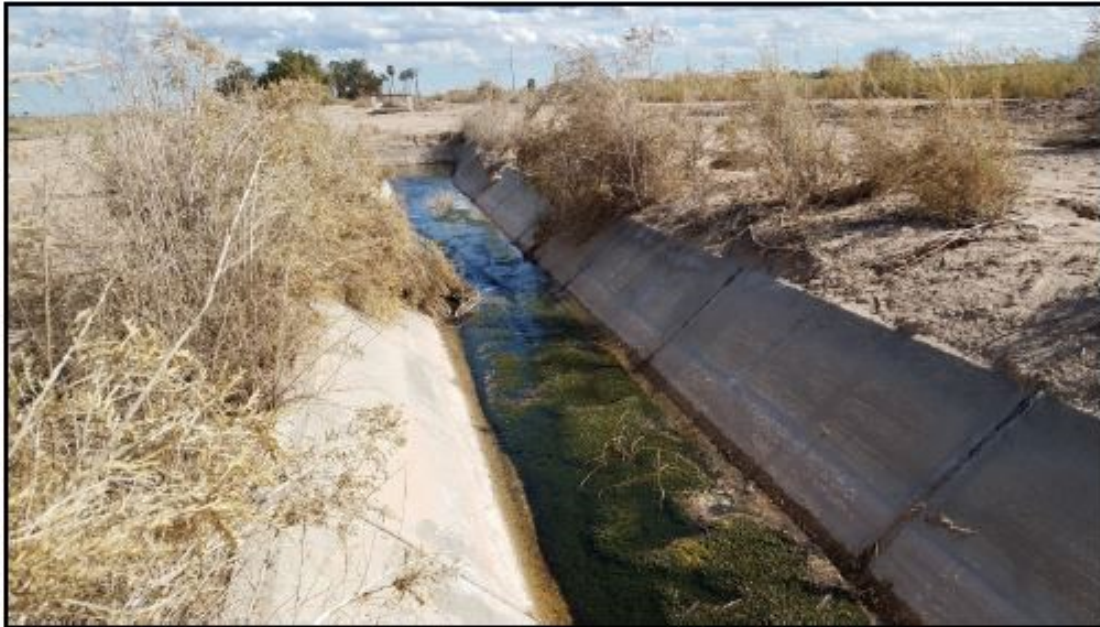
PHOTOGRAPH 5 View of East-west Concrete-lined Channel North of the Westside Canal, Facing East.
