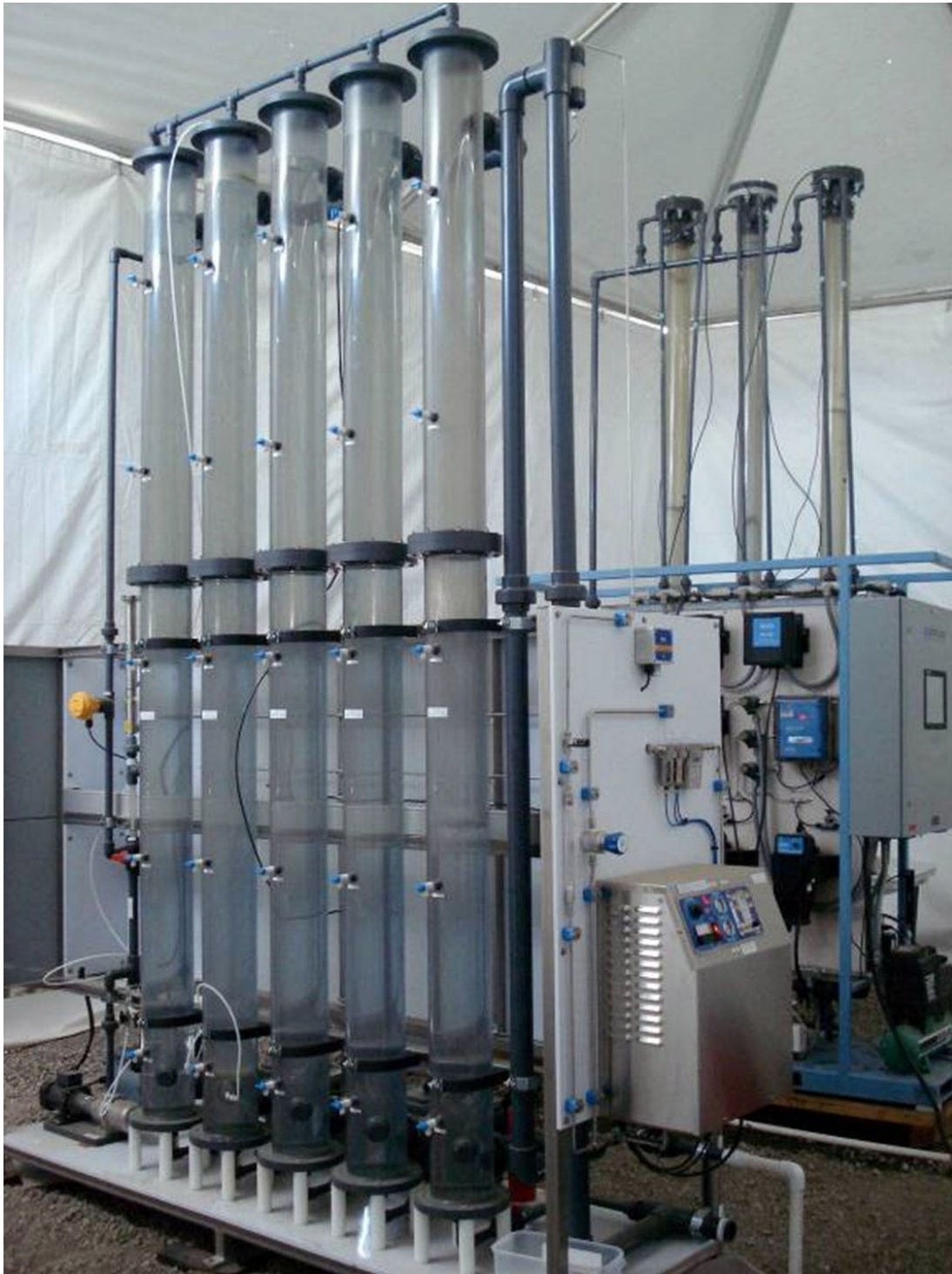
Figure 4 INTUITECH OZONE MODULE Z100 SET UP ON SITE AT BOLLMAN WTP CALIFORNIA DEPARTMENT OF WATER RESOURCES CALIFORNIA DEPARTMENT OF PUBLIC HEALTH
