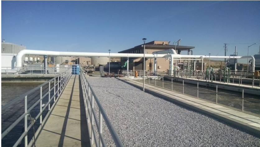
Main regional plant aeration basin in operation - VVWRA photo
