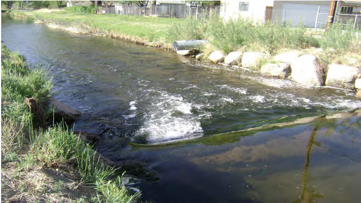
Photo 7-1 Concrete encased clay pipe submerged in water at a canal crossing. City of Bishop planned to replace this 15-inch clay pipe with a new 18-inch plastic pipe (more information contained in Section 7.5.3). Photo credit: John Morales/Lahontan Water Board
