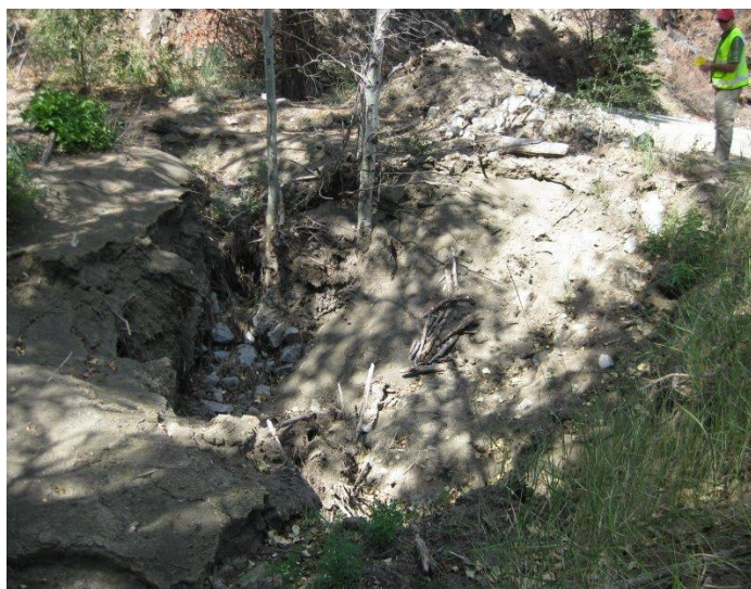
Culvert under Wolf Creek Road which was buried by the debris flow and subsequently caused flooding and erosion of the road bank and road shoulders
