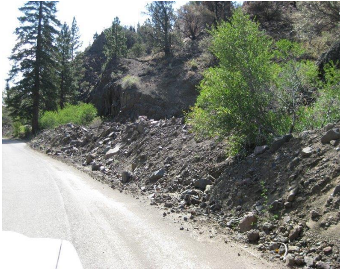
Accumulated debris along Wolf Creek Road piled in preparation for hauling
