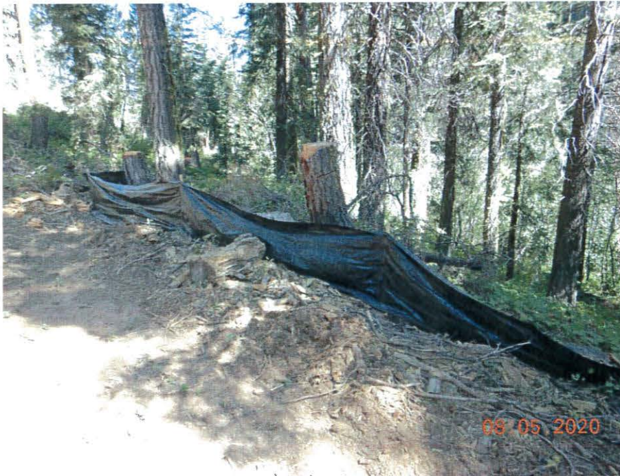
Photo 10. Downslope perimeter sediment control BMP.
