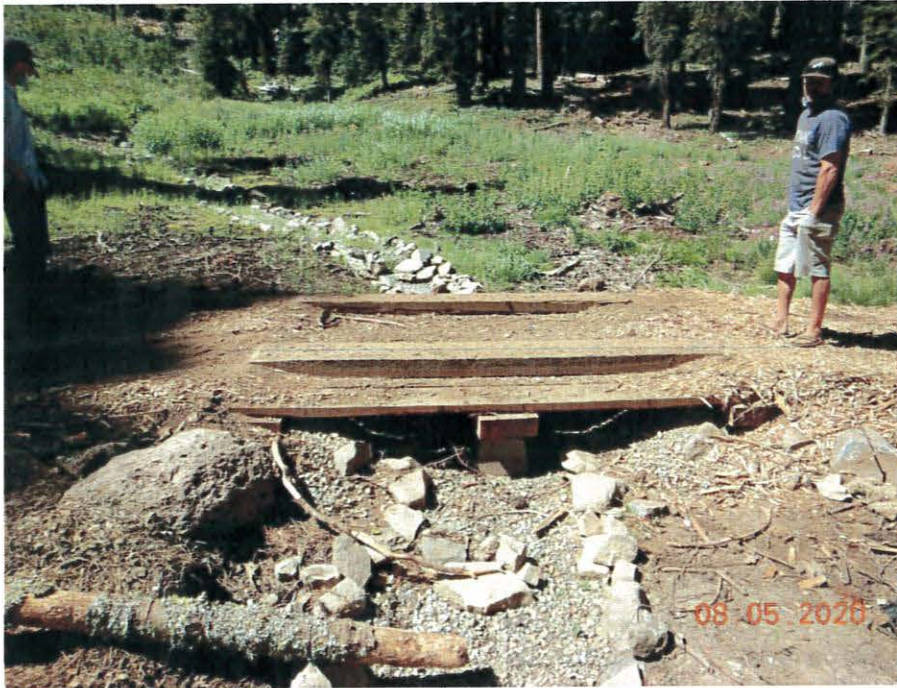
Photo 14: Permanent watercourse crossing.
