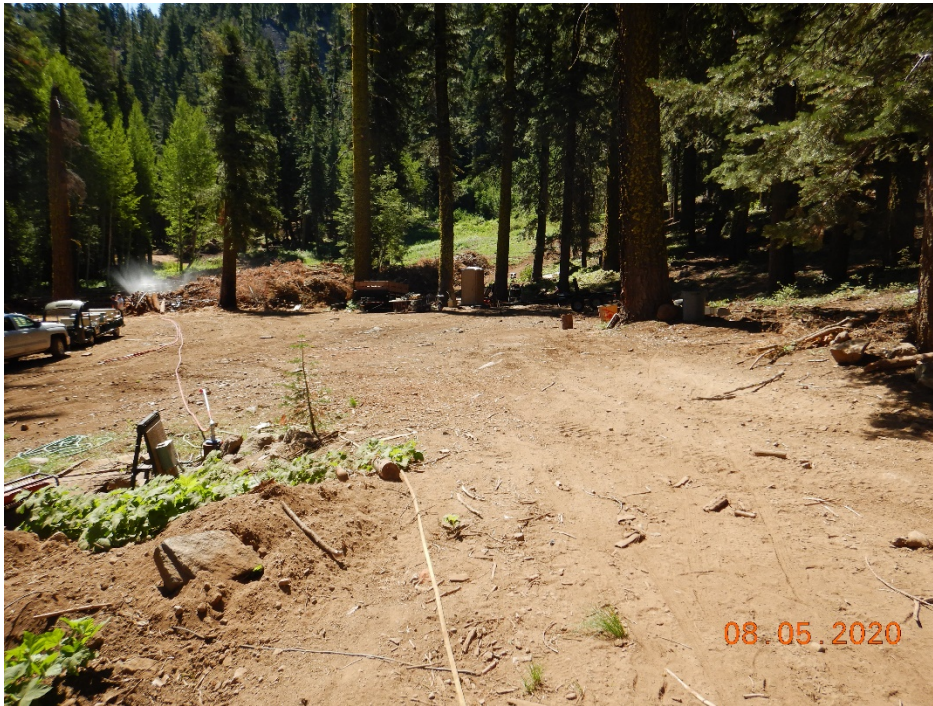
Photo 1. General site view showing recently cleared open area, windrowed soil and rock, slash pile, and small log deck.
