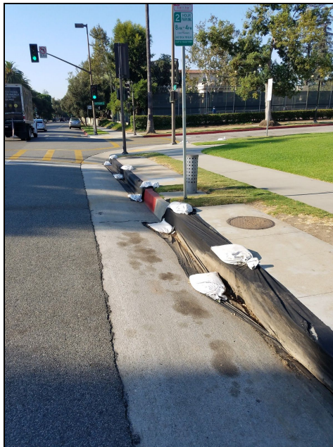
Figure 9. Covered catch basins along the Public/Educational Study route, on the corner of Hill and San Pasqual, preventing trash from being swept into them
