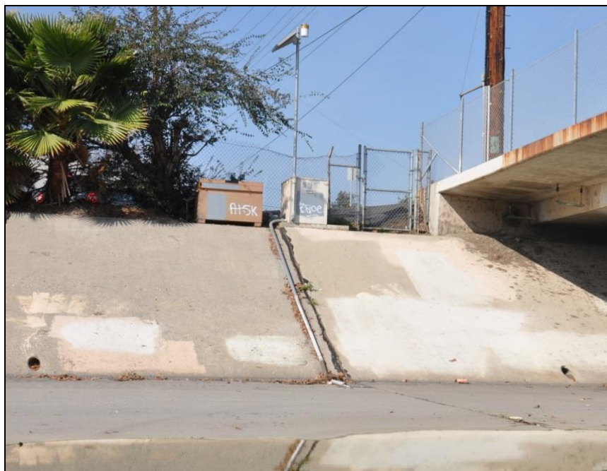
Figure 7: Stearns Street Mass Emission Station
