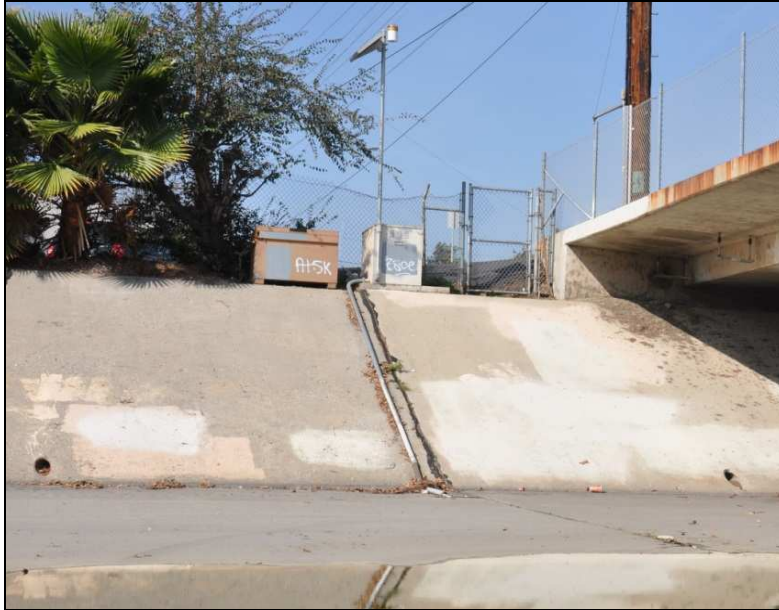
Figure 7: Stearns Street Mass Emission Station
