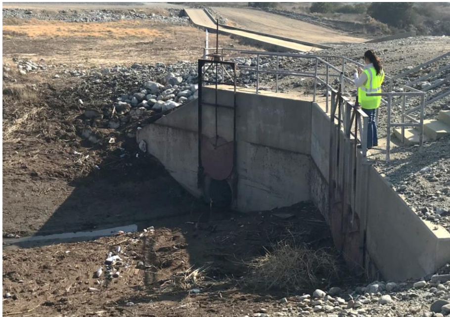
Figure 5. Basin 3E Outlet Gate Values with 48-Inch CMP Pipes
