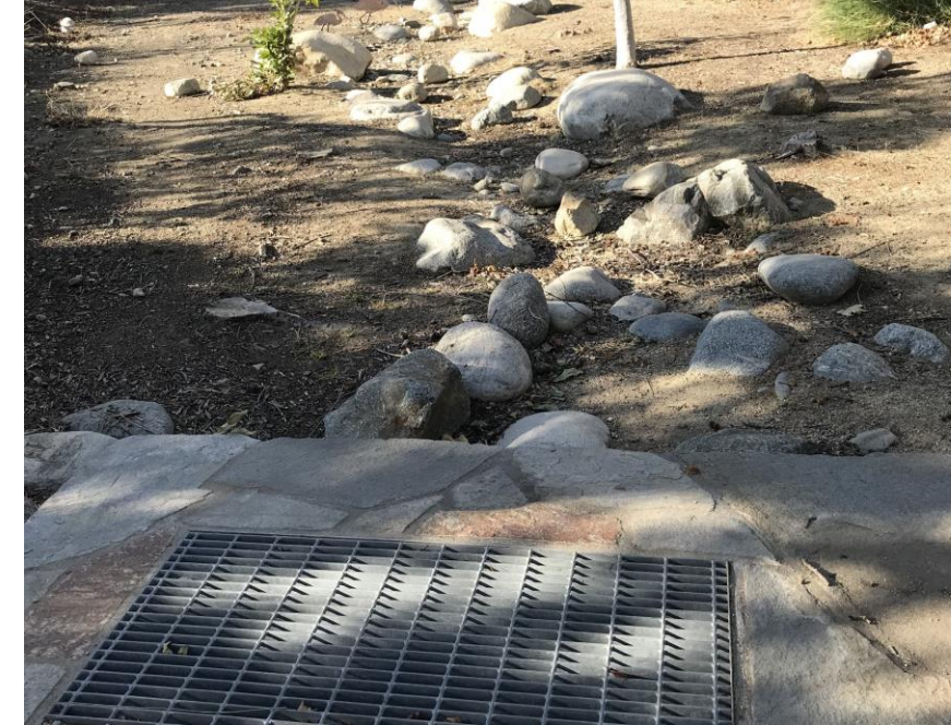
Close Up of Existing Grate Inlet (Circled in Red to Left) from Natural Channel to SD (from SE looking NW)
