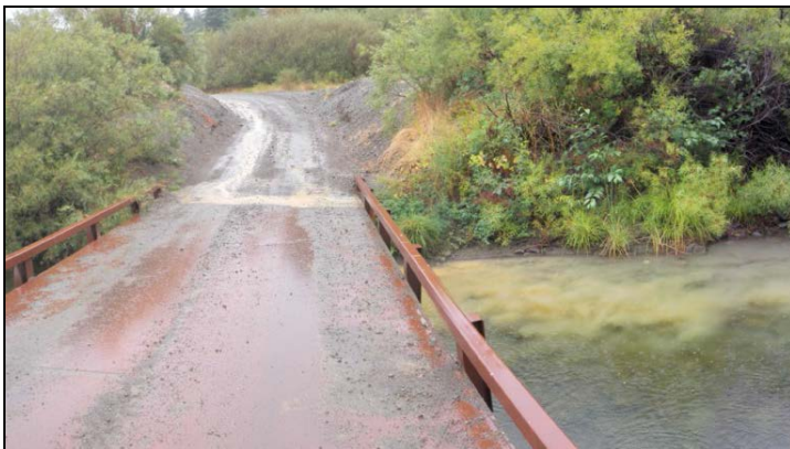
Weaver et al. 2014. Figure 21. Road approaches to bridges are often hydrologically connected. This through-cut approach to a temporary bridge drains directly into the stream.
