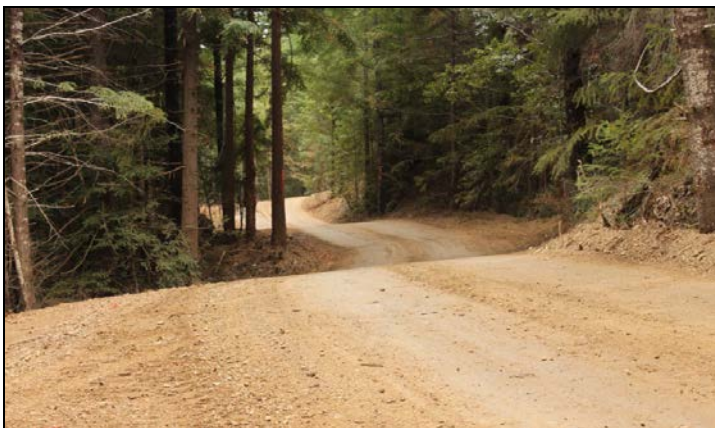
Weaver et al. 2014. Figure 28. Well built, outsloped road displaying minimum cut, smooth free draining surface, and no outside berm. The road contours with the topography and its rolling grade and rolling dips disperse surface runoff.
