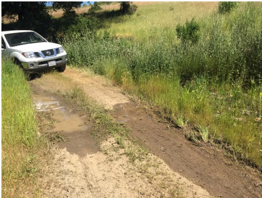
PWA Site #10. Overgrown vegetation preventing proper road drainage. (May 2017)
