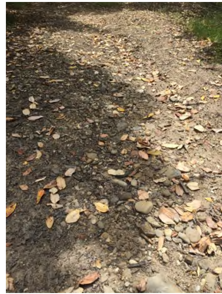
PWA RD #37 further down road, rill hits gravelly native road layer before exiting at RD #38 (May 2016)
