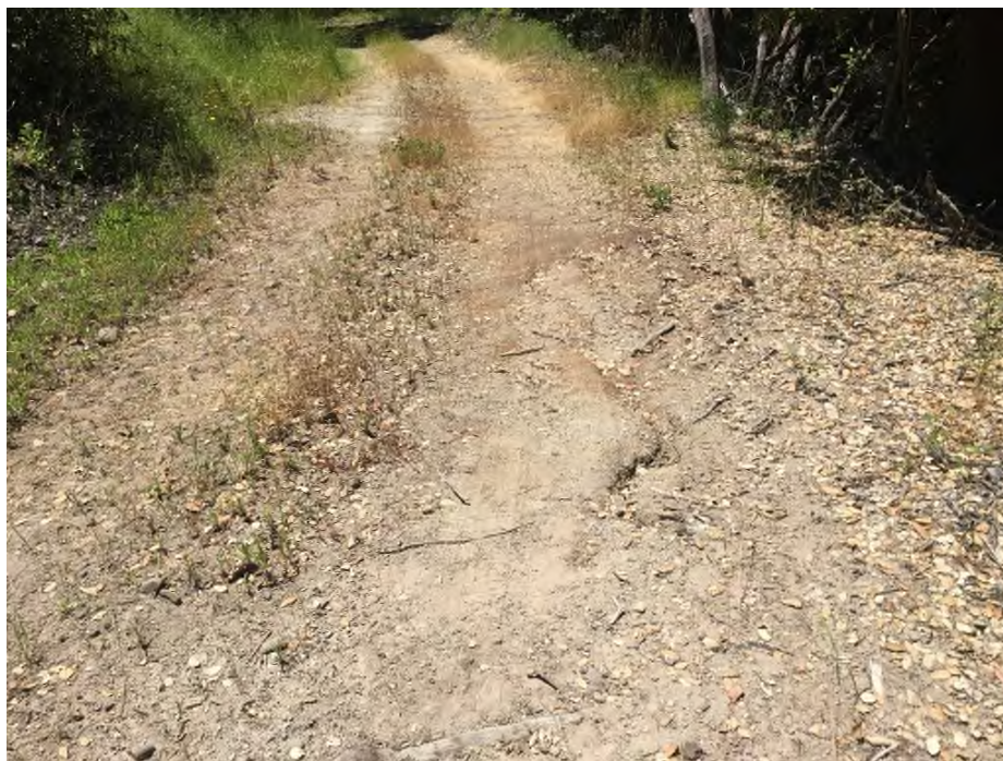
PWA RD #37 small rill which exits road bed to right (May 2017)
