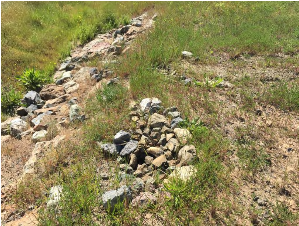
PWA Site 7.2c Rock armor treatment for holes above rock armor one of two sets (May 2017)
