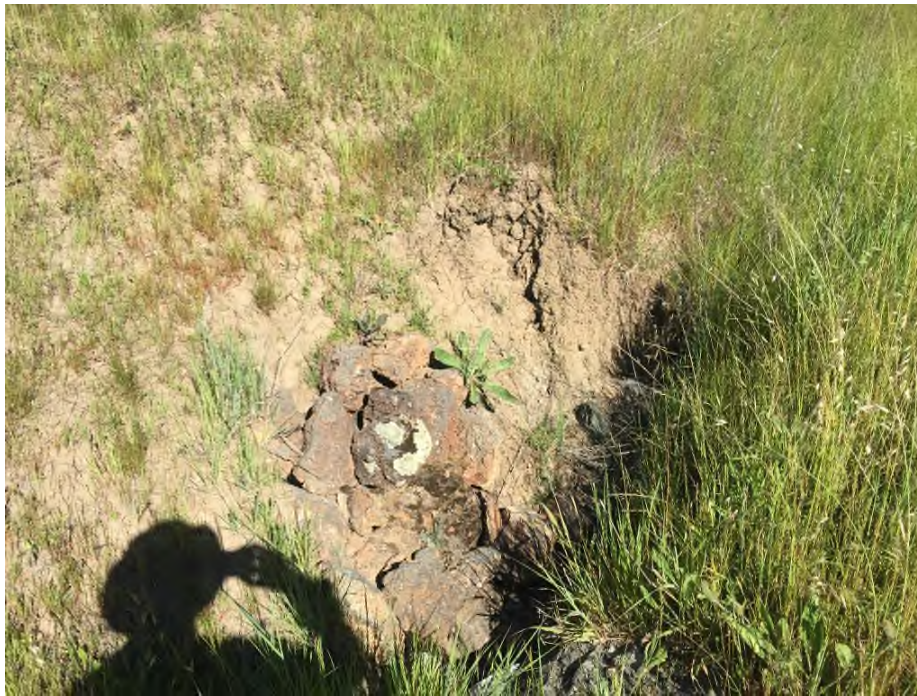
PWA RD #46.1 A 1-foot vertical headcut and 2-foot wide scour area has developed in the ditch above the DRC inlet (May 2017)
