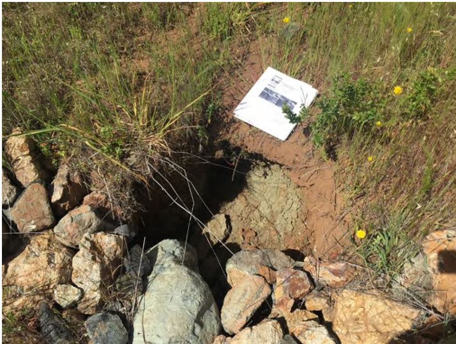
PWA Site #8.1 Grade Control Structure Headcut (May 2016)
