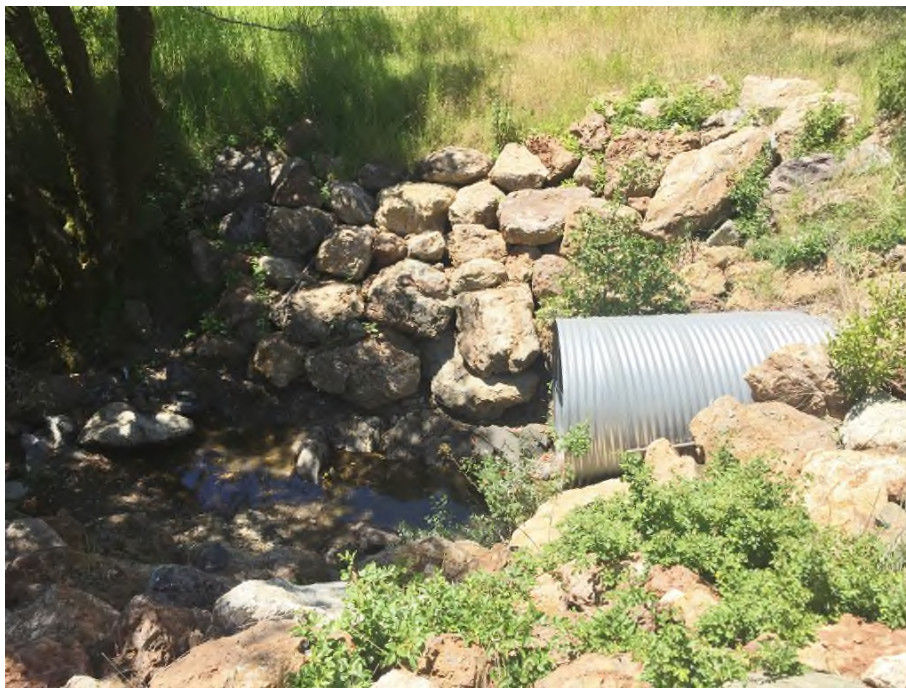
PWA Site #6 outlet (May 2017). Repair work on 9/26/2015 still holding up.
