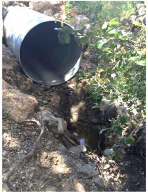
PWA Site #5 scour pool (May 2016)
