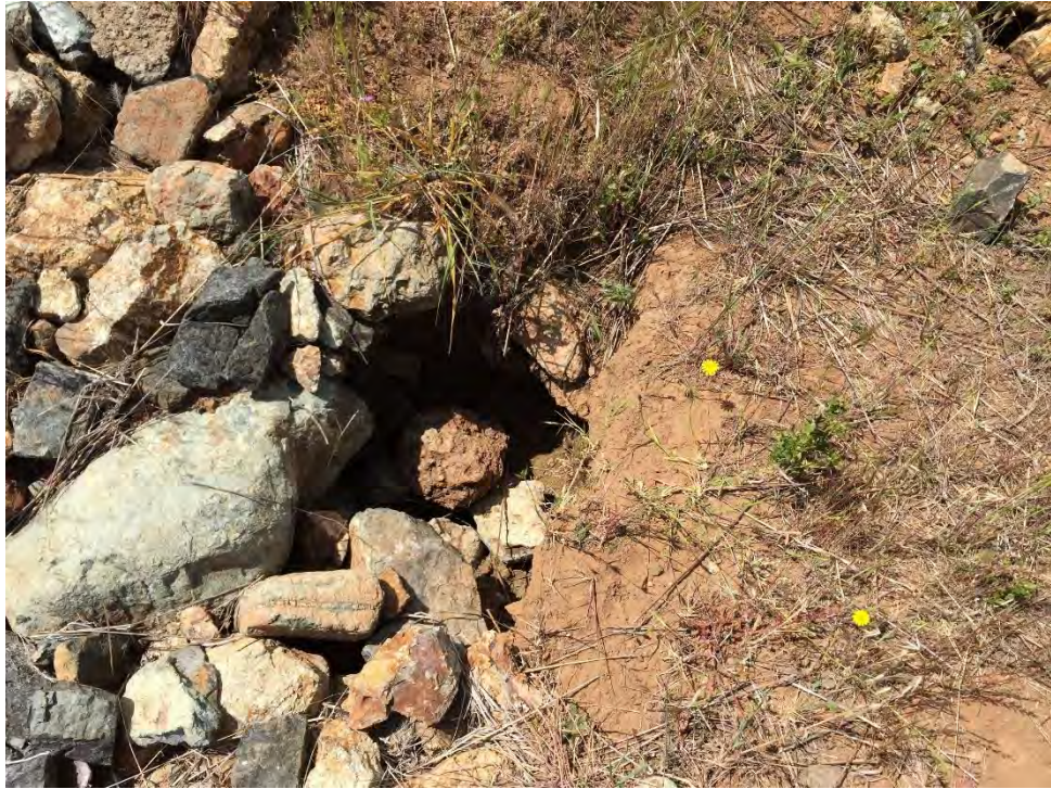
PWA Site #8.1 Grade Control Structure Headcut (May 2015)
