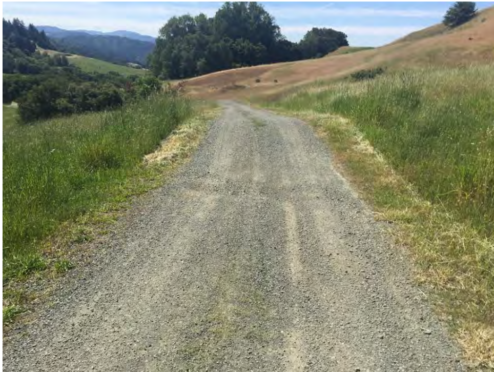
PWA RD1: Shallow depression (May 2016)
