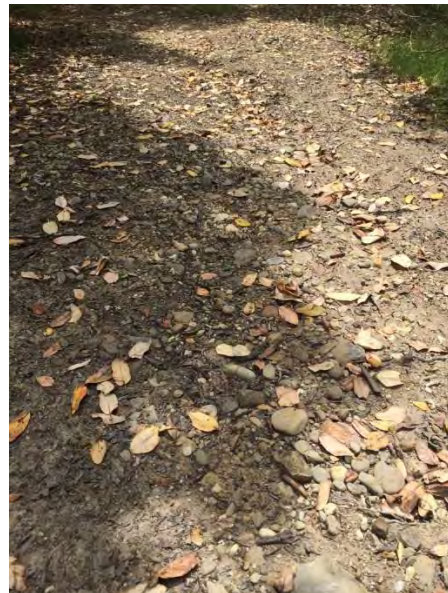
PWA RD #37 further down road, rill hits gravelly native road layer before exiting at RD #38 (May 2016)
