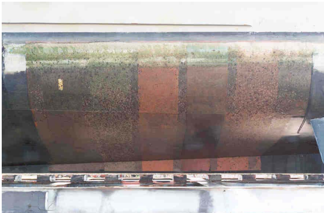
Figure 9: Port side midships test strips on HMAS TOWNSVILLE at completion of trial after 31 months
