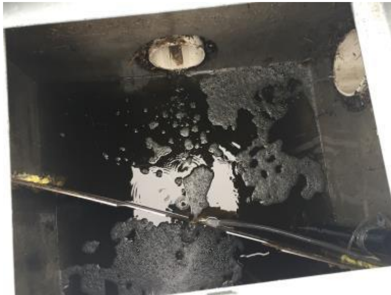
Figure 2-8 Influent autosampler sample at pretreatment chamber of Parking Lot 5 MWS No. 2
