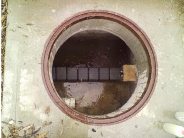
Figure 2-7 Effluent grab sample location at discharge chamber of Parking Lot 5 MWS No. 2
