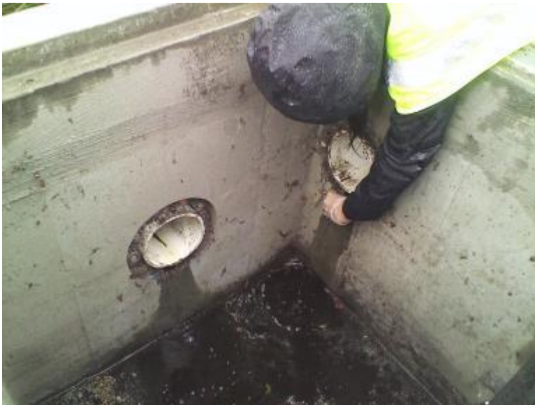
Figure 2-6 Influent grab sample at pretreatment chamber of Parking Lot 5 MWS No. 2
