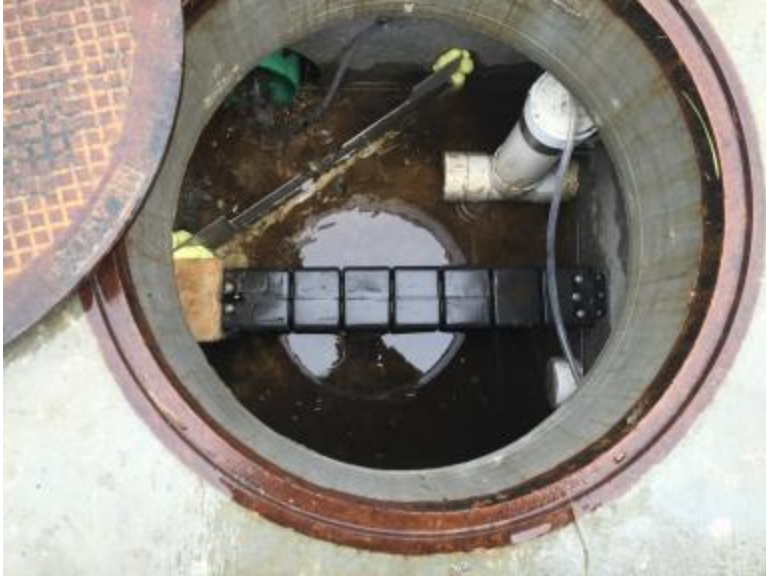
Figure 2-9 Effluent autosampler sample at discharge chamber of Parking Lot 5 MWS No. 2
