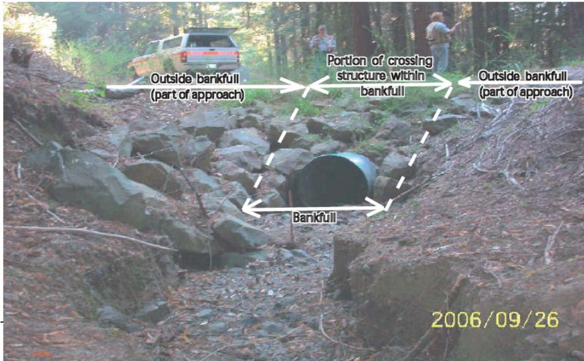
Figure 12. The fill material from the hinge points to the dashed lines is considered part of the approach. The crossing itself is only the area between the dashed lines.
