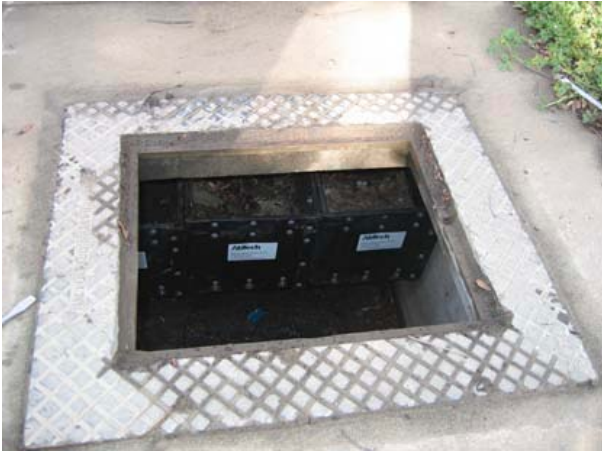
Filter installed in Catch Basin
