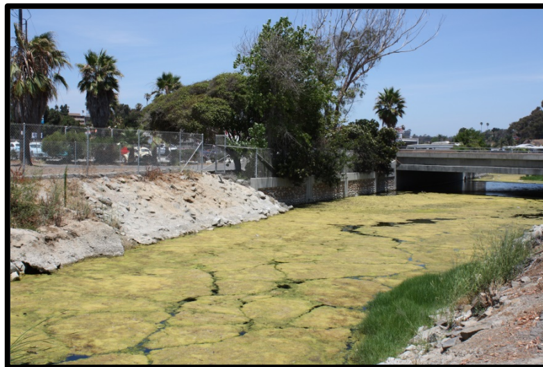
FIGURE 3 VIEW OF SHOTCRETE-LINED SECTION OF LOMA ALTA CREEK View to east (upstream). Photograph taken south of Pacific Coast Highway.
