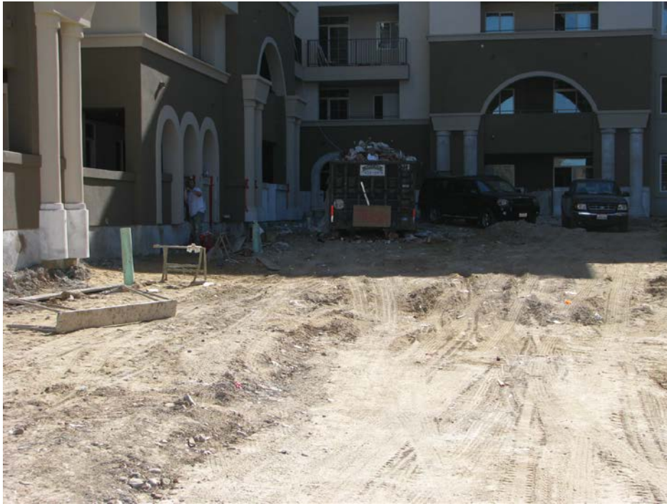
Figure 7. Site interior with overflowing waste bin
