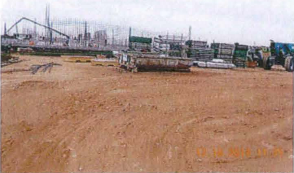
#23 Cover WASHOUT PRIOR TO RAIN.
