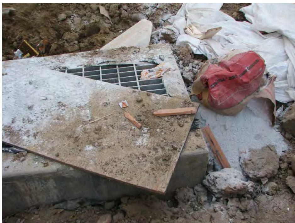
Figure 24. Storm drain littered with construction debris
