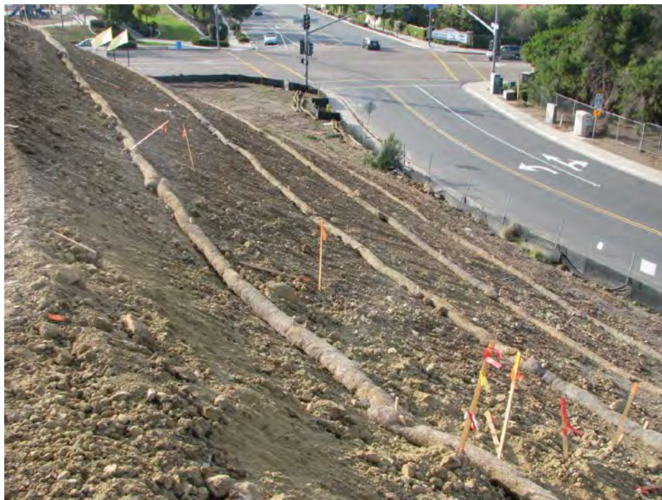
Figure 9. Slope on north side with no erosion control
