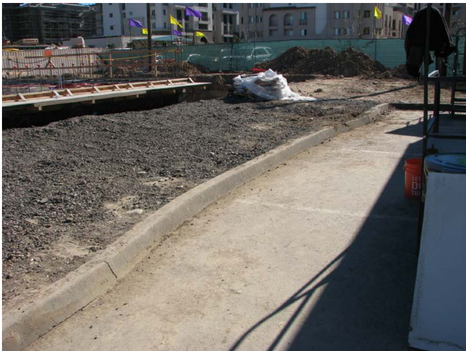
Figure 8. Curb in front of trailer; cigarettes have been swept up
