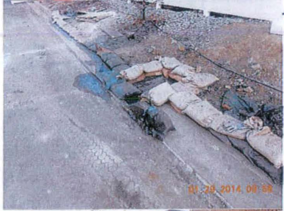
#11 Replace broken bags
