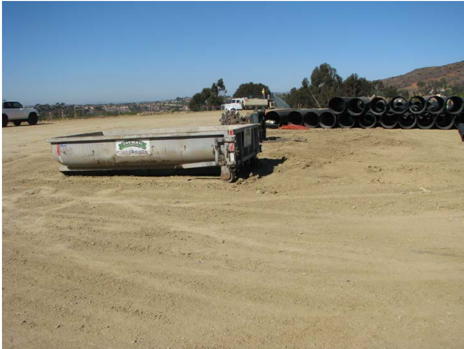
Figure 9. Leaking concrete waste bin has been replaced
