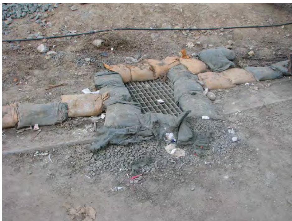
Figure 22. Broken gravel bags
