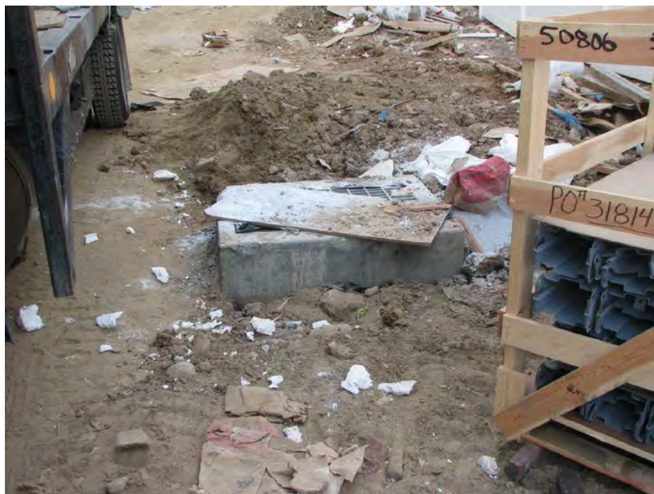
Figure 23. Storm drain littered with construction debris
