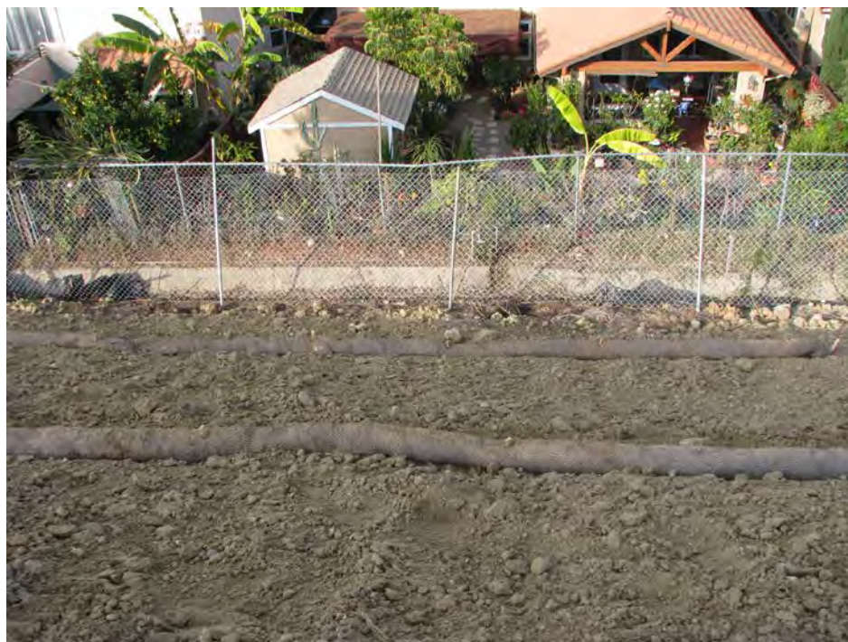
Figure 13. Damaged silt fence
