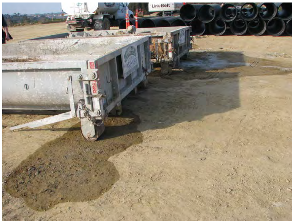
Figure 7. Leaking concrete washouts
