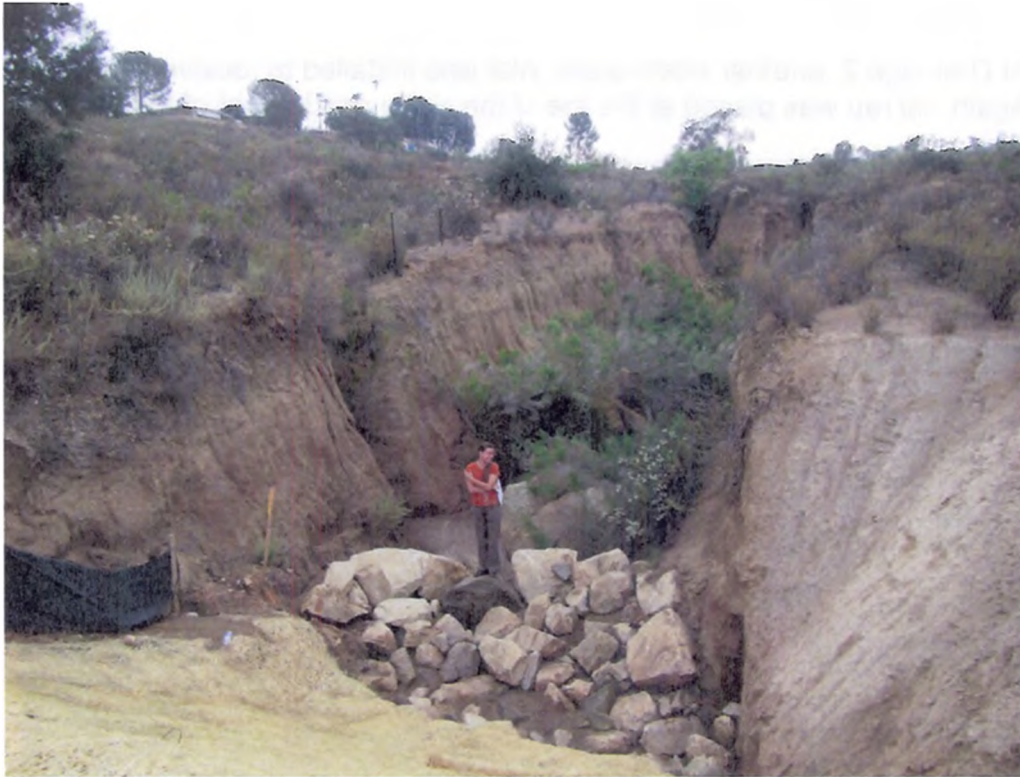
Photo 2: Looking down from the top of the road knuckle into Drainage 1. Melanie Tymes of the Army Corps is approximately 5'4" in height.
