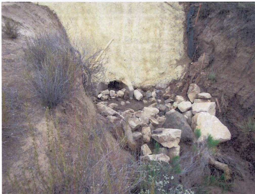
Photo 3: Storm water inlet structure installed at the base of the fill in Drainage 1.
