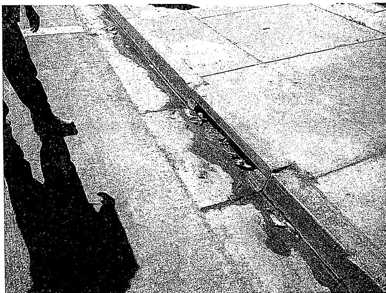
2. Dirty street and gutter at the curb outlet from the school's storm drain system.
