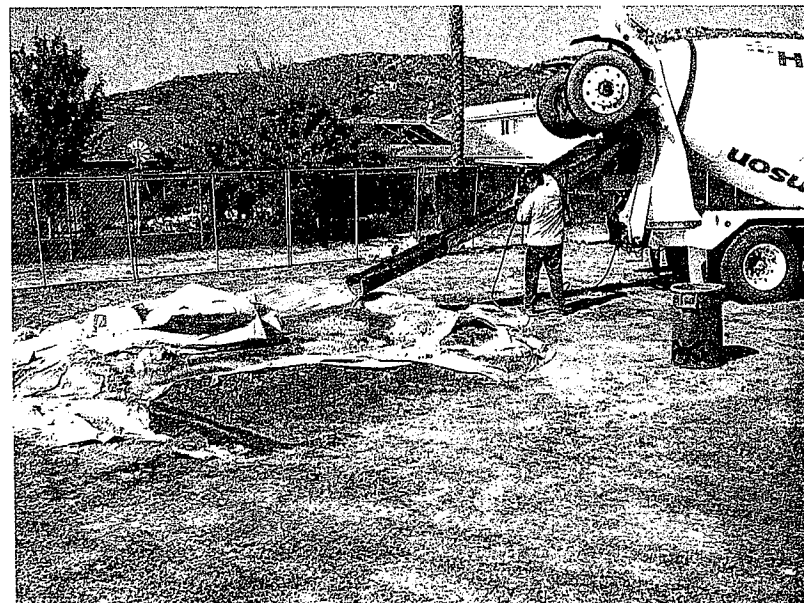
6. Concrete washout was continuing to be used although inadequate.
